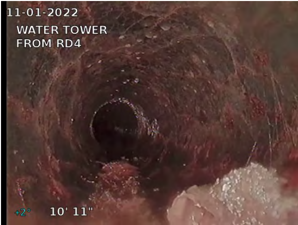
9, 00:00:50, 10.92ft Crack Multiple from 9 o'clock to 3 o'clock
