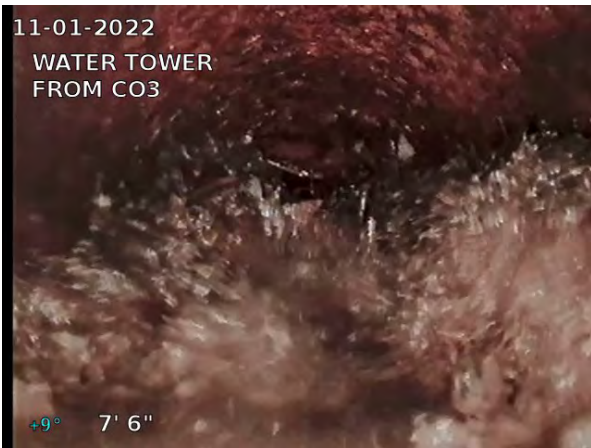
7, 00:01:01, 7.50ft Obstruction Other, 100% of cross sectional area from 12 o'clock to 12 o'clock / BLOCKAGE - ROOTS, LEAVES, SEDIMENT, MISC DEBRIS
