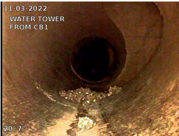
3, 00:00:34, 20.58ft Tap Factory Made at 3 o'clock, dia/height: 8inch
