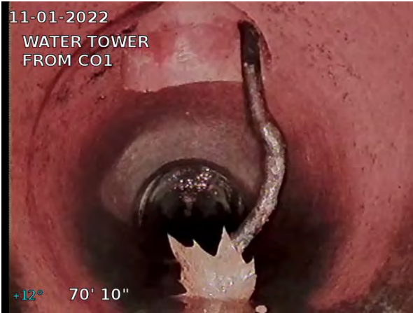
9, 00:02:47, 70.84ft Obstruction Through Connection, 5% of cross sectional area at 12 o'clock / SMALL BRANCH WEDGED AT CLEANOUT
