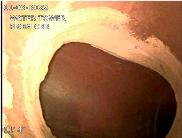
5, 00:00:44, 11.33ft Tee Connection / TIES INTO MAIN FROM CB1
