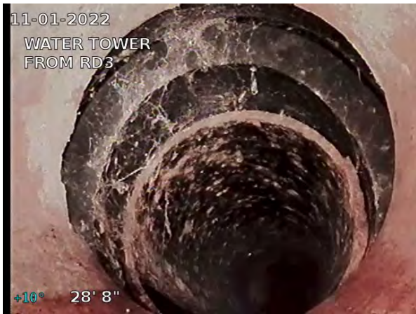
11, 00:02:01, 28.67ft Miscellaneous Shape or Size Change, dia/height: 6inch / REDUCES TO 6 INCH PIPE
