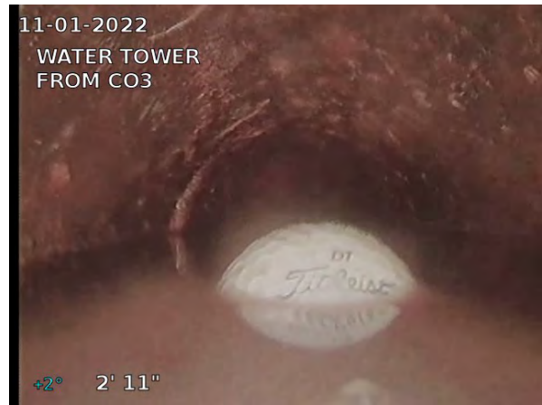
4, 00:00:21, 2.92ft Deposits Settled Fine, 25% of cross sectional area from 4 o'clock to 8 o'clock
