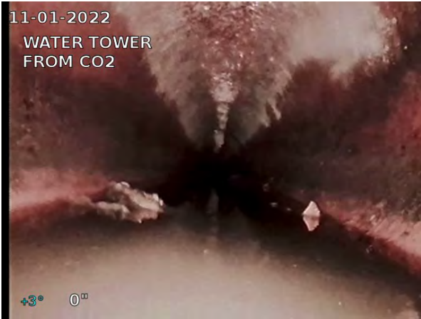
1, 00:00:00, 0.00ft Cleanout Mainline / CO2
