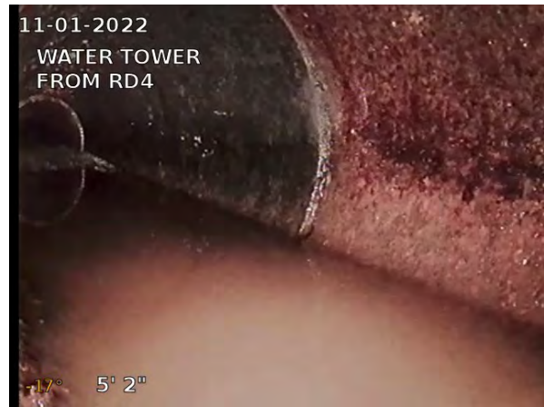
4, 00:00:25, 5.16ft Miscellaneous General Observation / WYE LEFT INTO 6 INCH MAIN
