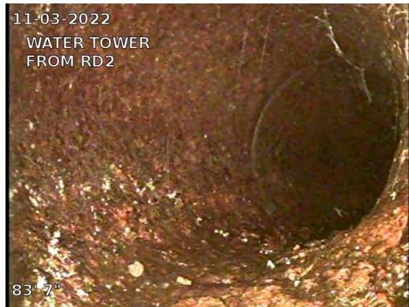
8, 00:02:18, 83.58ft Miscellaneous General Observation / LINE ANGLES RIGHT
