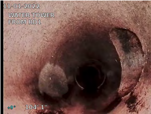
9, 00:04:24, 104.08ft Tap Factory Made at 3 o'clock, dia/height: 4inch
