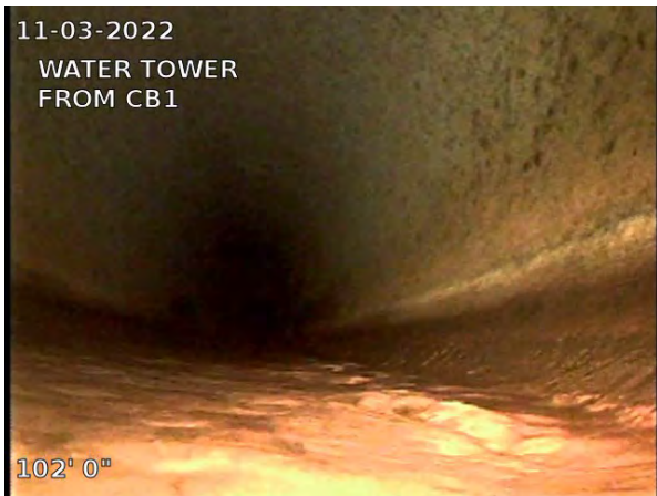
11-03-2022 WATER TOWER FROM CB1 102' 0" 11, 00:03:52, 102.00ft Miscellaneous Survey Abandoned / CAMERA WOULD NOT PUSH FURTHER DUE TO FRICTION
