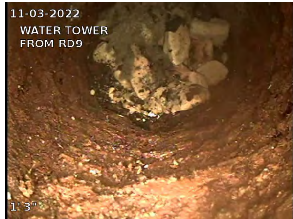
4, 00:00:35, 1.25ft Miscellaneous Survey Abandoned / RISER FILLED WITH STONES, CANNOT ENTER LINE
