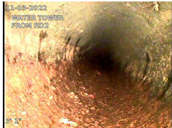
4, 00:00:22, 3.08ft Miscellaneous Shape or Size Change, dia/height: 6inch / 6 INCH MAIN
