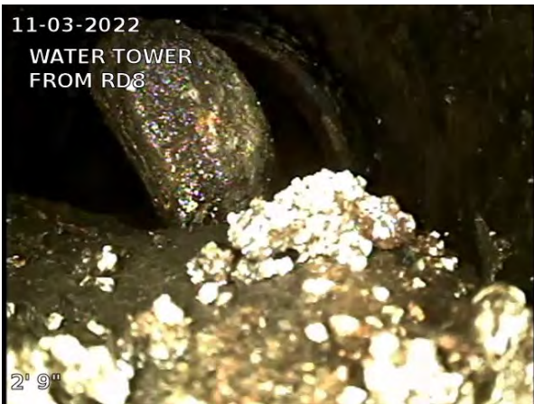
3, 00:00:10, 2.75ft Deposits Settled Other, 50% of cross sectional area from 3 o'clock to 9 o'clock / SEDIMENT AND STONE
