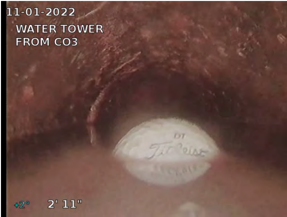
5, 00:00:21, 2.92ft Obstruction Other, 10% of cross sectional area at 6 o'clock / GOLF BALL
