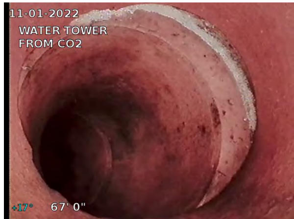
4, 00:02:02, 67.00ft Miscellaneous General Observation / LINE ANGLES LEFT
