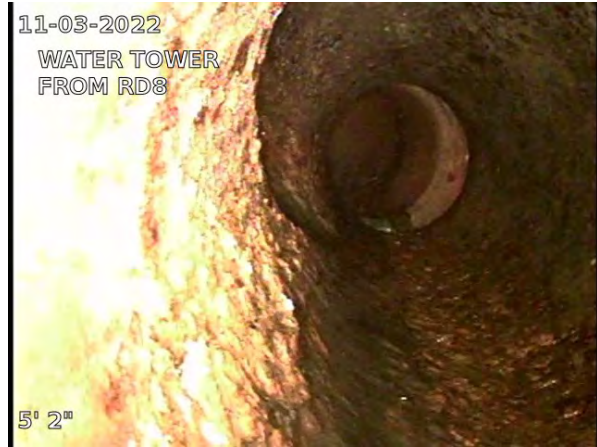
6, 00:00:33, 5.16ft Tap Factory Made at 10 o'clock, dia/height: 4inch
