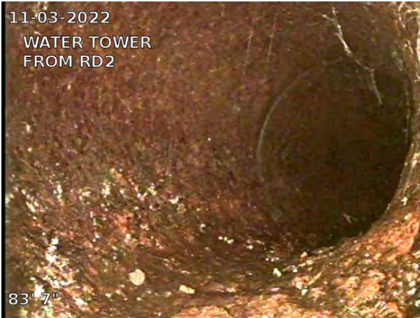
9, 00:02:18, 83.58ft Deposits Settled Fine, 5% of cross sectional area from 5 o'clock to 7 o'clock, within 8 inch, Finish
