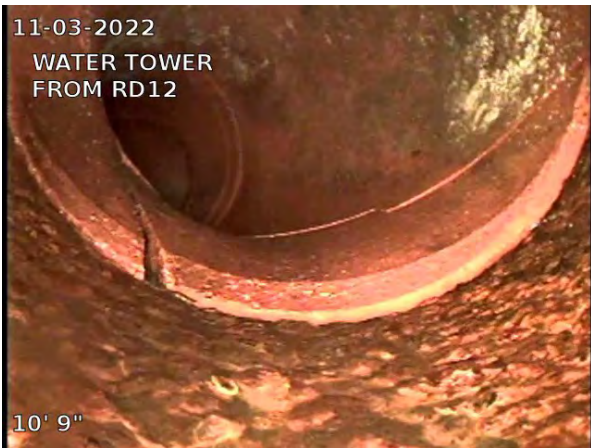
7, 00:00:34, 10.75ft Fracture Circumferential from 4 o'clock to 8 o'clock
