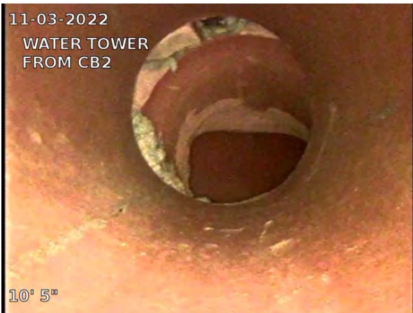
3, 00:00:24, 10.42ft Joint Separated Large, 1Inch, 1Inch / SEPERATION AT JOINT
