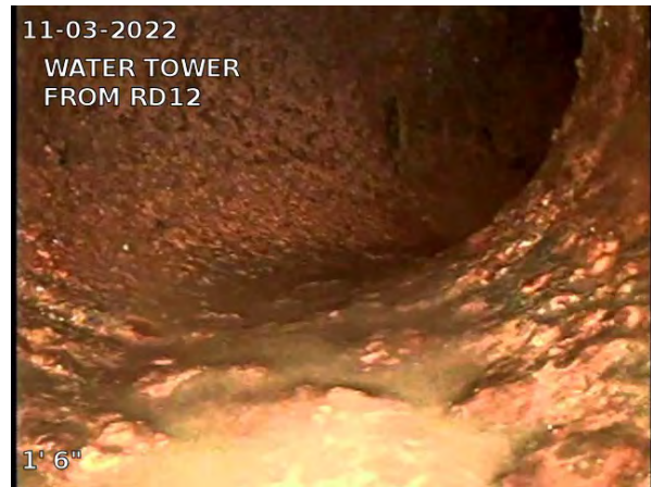
4, 00:00:09, 1.50ft Miscellaneous General Observation / LINE ANGLES LEFT
