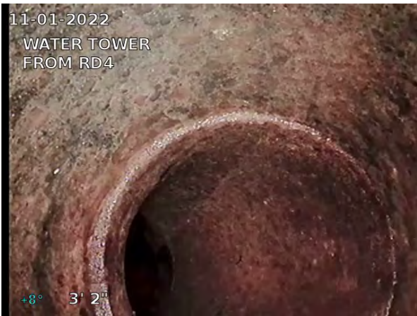
3, 00:00:14, 3.16ft Miscellaneous General Observation / LINE ANGLES LEFT
