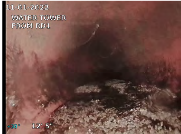
6, 00:01:02, 12.42ft Miscellaneous Shape or Size Change, dia/height: 6inch / 6 INCH MAIN
