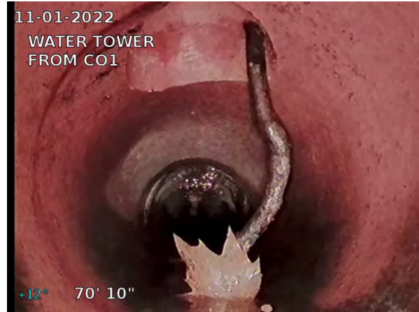
10, 00:02:47, 70.84ft Cleanout Mainline / CO2
