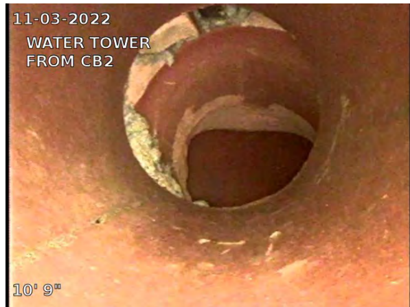
4, 00:00:24, 10.42ft Joint Separated Large, 1Inch, 1Inch / SEPERATION AT JOINT
