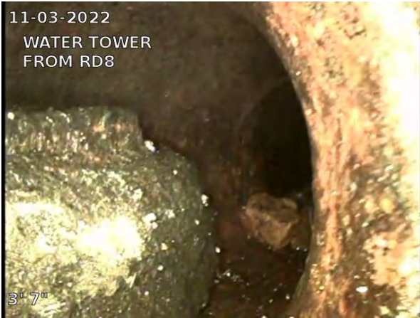
5, 00:00:20, 3.58ft Miscellaneous General Observation / LINE ANGLES RIGHT
