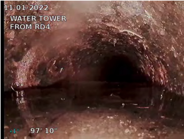
17, 00:03:56, 97.84ft Deposits Settled Fine, 25% of cross sectional area from 4 o'clock to 8 o'clock
