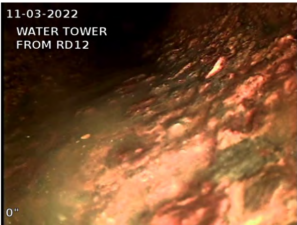
3, 00:00:00, 0.00ft Miscellaneous General Observation / TRAP AT BOTTOM OF RISER, RUN BEGINS AFTER CAMERA HAS PASSED THROUGH TRAP
