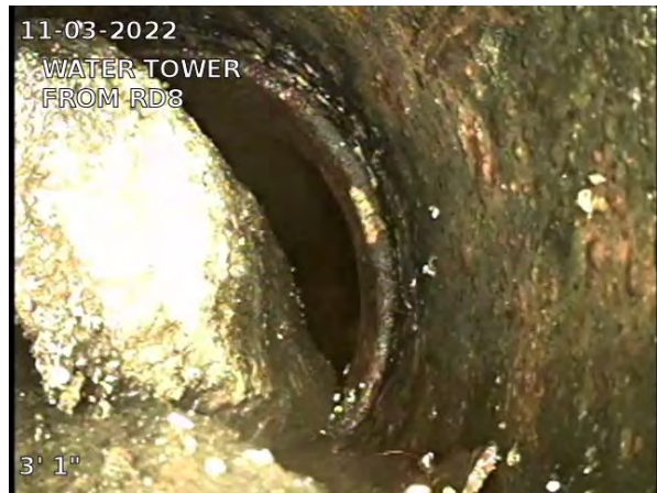
4, 00:00:10, 2.75ft Deposits Settled Other, 50% of cross sectional area from 3 o'clock to 9 o'clock / SEDIMENT AND STONE
