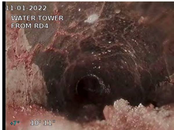
8, 00:00:50, 10.92ft Crack Multiple from 9 o'clock to 3 o'clock
