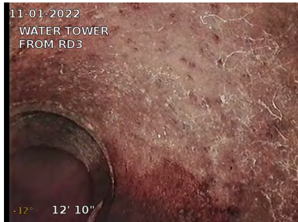
4, 00:00:41, 12.84ft Miscellaneous General Observation / WYE LEFT
