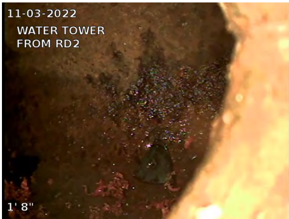
3, 00:00:14, 1.67ft Miscellaneous General Observation / WYE LEFT INTO 6 INCH MAIN
