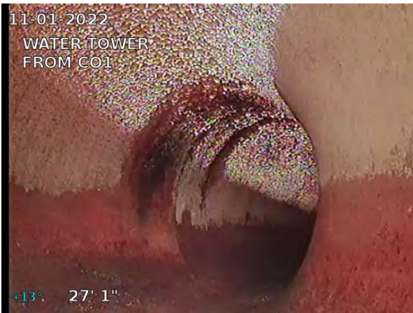
3, 00:00:51, 27.08ft Miscellaneous General Observation / LINE ANGLES RIGHT
