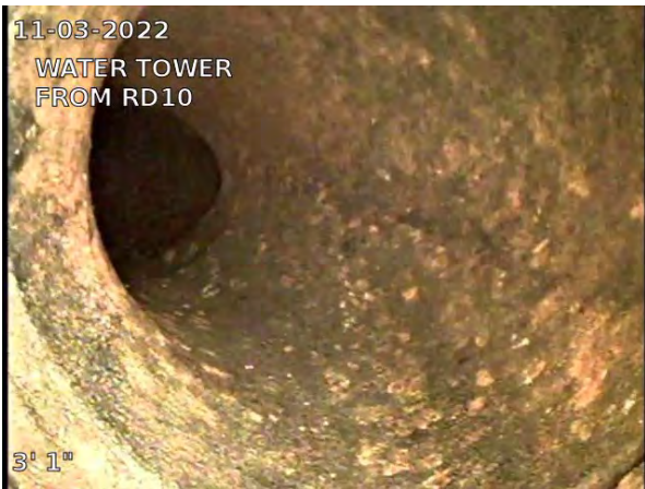
3, 00:00:08, 3.08ft Miscellaneous General Observation / WYE LEFT
