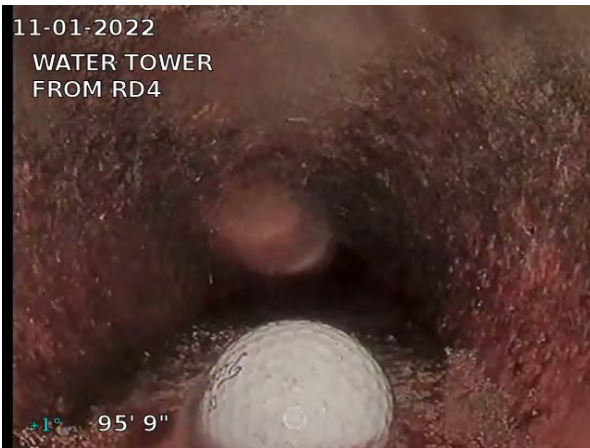
15, 00:03:50, 95.75ft Obstruction Other, 10% of cross sectional area at 6 o'clock / GOLF BALL
