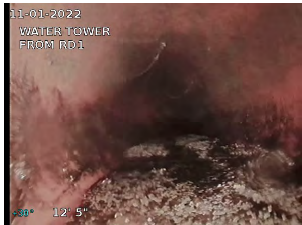
4, 00:01:02, 12.42ft Miscellaneous General Observation / TIES INTO MAIN
