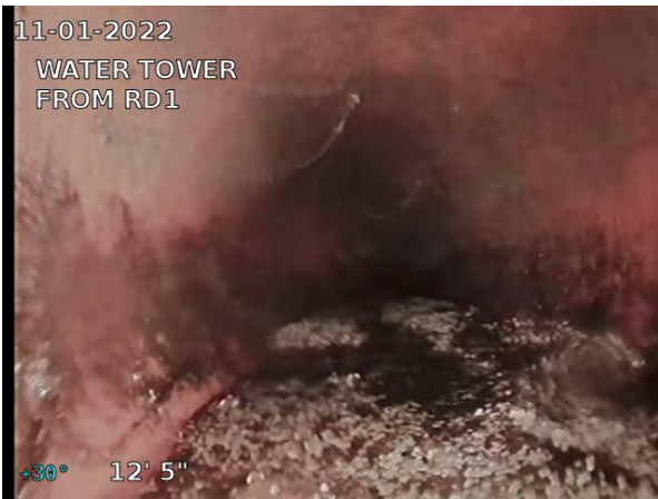
7, 00:01:02, 12.43ft Deposits Settled Fine, 5% of cross sectional area from 5 o'clock to 7 o'clock, within 8 inch, Start
