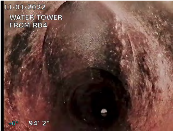
13, 00:03:37, 94.16ft Tap Factory Made at 12 o'clock, dia/height: 4inch / CO3
