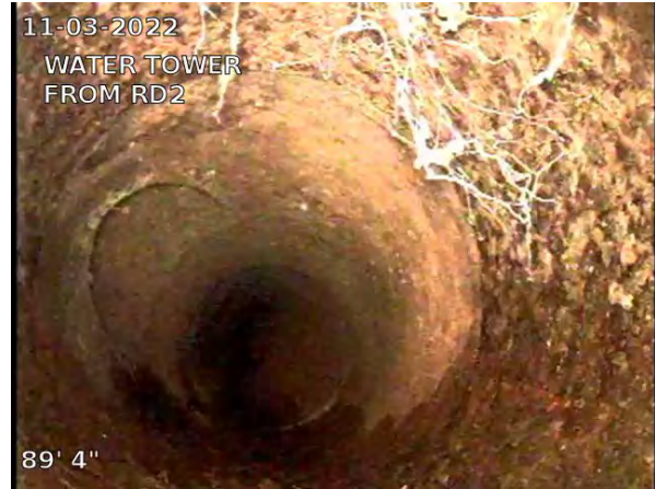
10, 00:02:46, 89.33ft Tap Factory Made at 9 o'clock, dia/height: 4inch
