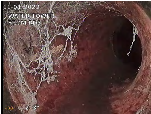
3, 00:00:09, 2.67ft Miscellaneous General Observation / LINE ANGLES RIGHT
