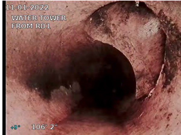
10, 00:04:38, 106.16ft Tap Factory Made at 2 o'clock, dia/height: 4inch
