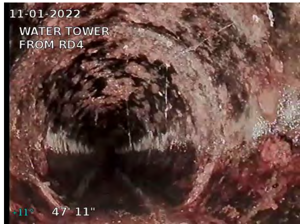
12, 00:02:11, 47.92ft Deposits Settled Fine, 10% of cross sectional area from 5 o'clock to 7 o'clock, within 8 inch, Finish
