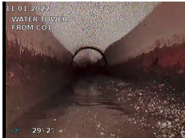
4, 00:01:01, 29.16ft Deposits Settled Fine, 5% of cross sectional area from 5 o'clock to 7 o'clock, within 8 inch, Start
