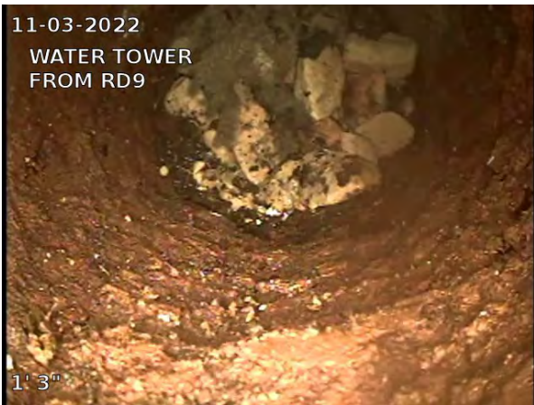
3, 00:00:34, 1.25ft Obstruction Rocks, 100% of cross sectional area from 12 o'clock to 12 o'clock / RISER FILLED WITH STONES
