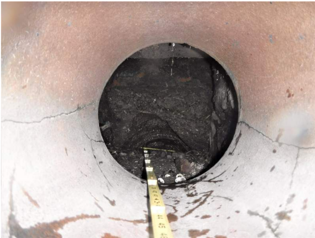
Photo 6: Collapsed and clogged outlet pipe at Sta. 11+10.
