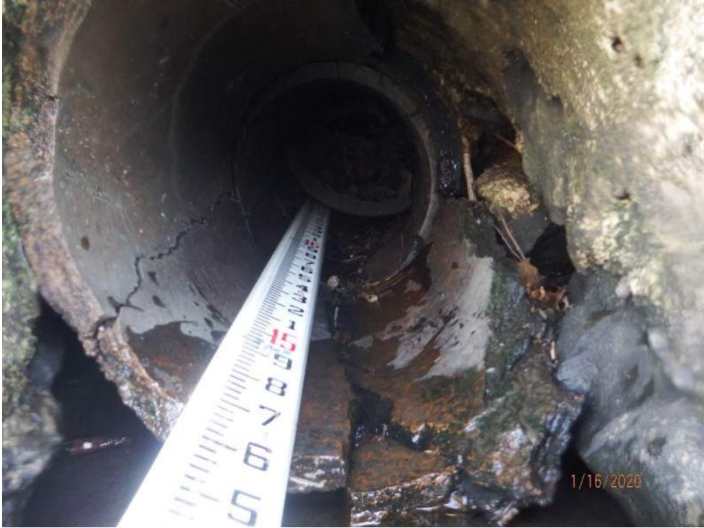
Photo 5: Collapsed weep hole at Sta. 0+48.
