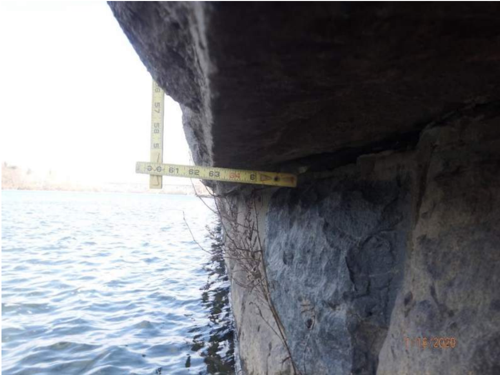
Photo 8: Top row of stones overhanging. (Station 9+50 Shown)
