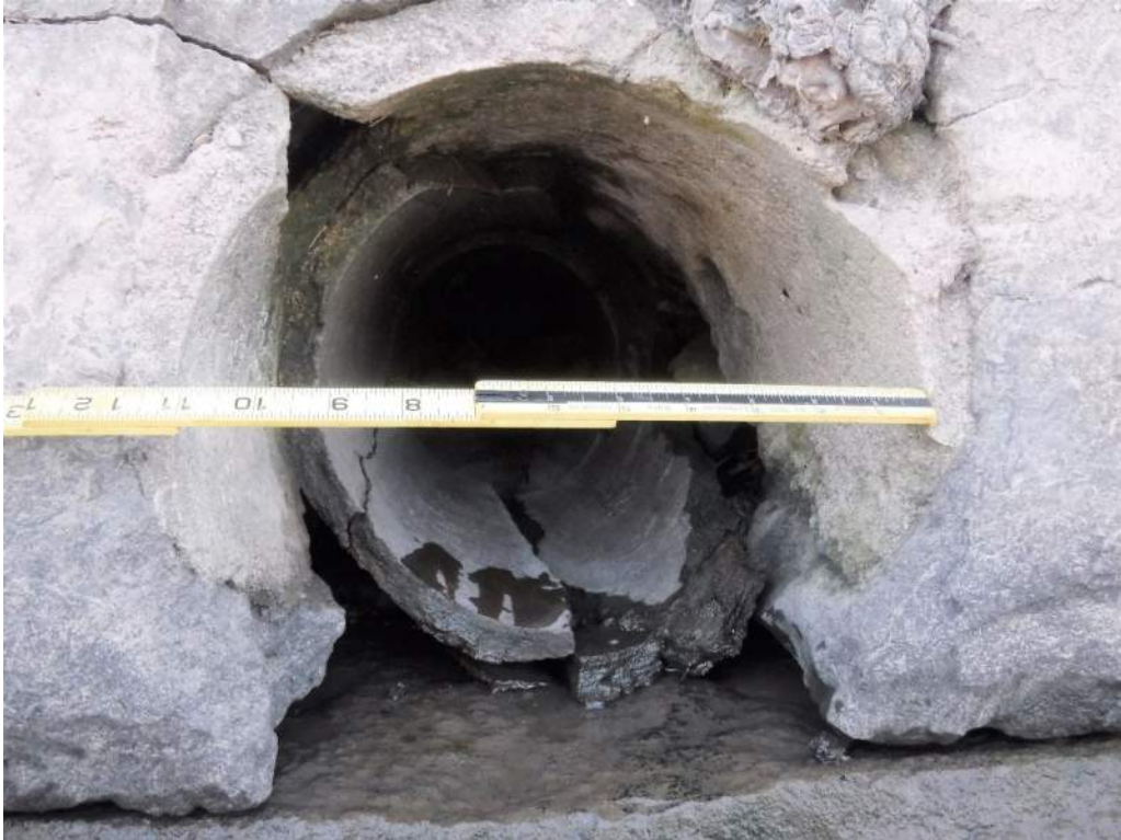
Photo 5: Collapsed outlet pipe at Sta. 0+60.
