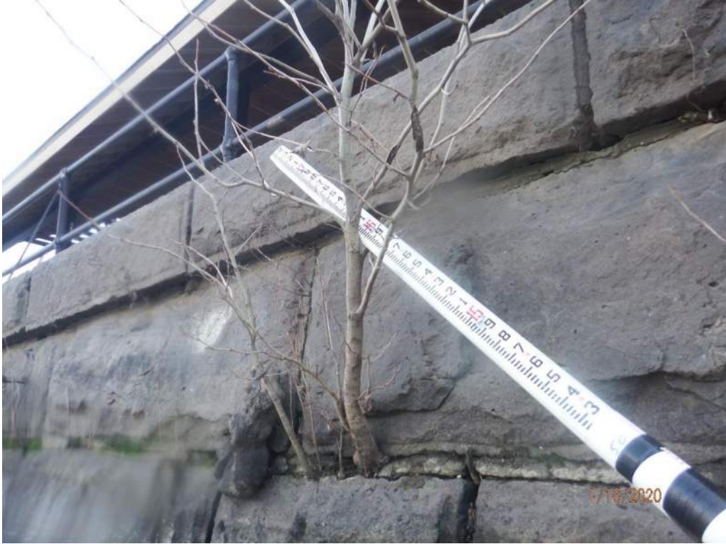
Photo 7: Typical vegetation growing in seawall.
