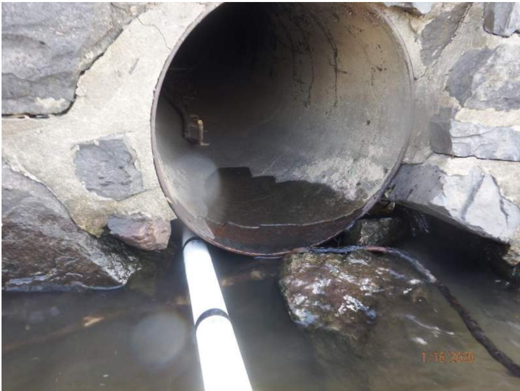
Photo 6: 2.1-foot void under outlet pipe at Station -5+80
