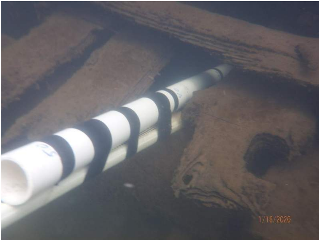
Photo 4: Area of undermining (Station 8+75 Shown)
