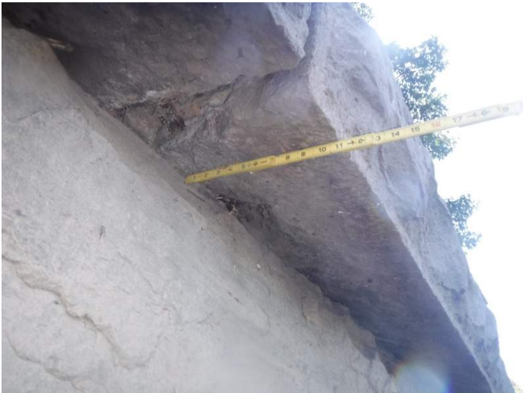
Photo 4: Overhang of top row of stone at Sta. 11+00.
