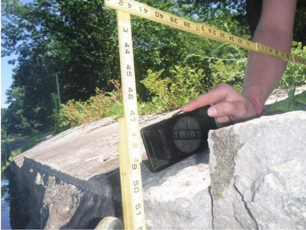
Photo 3: Rotation of top row of stone at Sta. 10+50.
