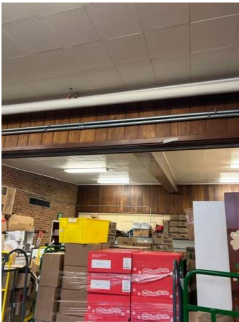
Fiberglass Pipe Insulation; Assumed Asbestos Pipe Insulation above Ceiling Tile/Plaster Ceiling System
