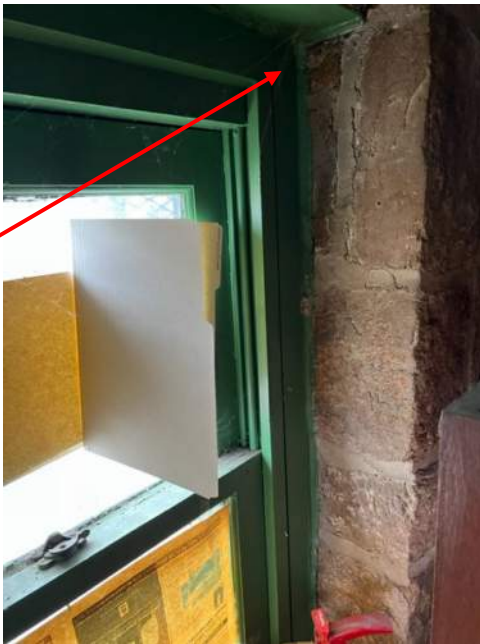
Asbestos Window Caulk in Small Office
