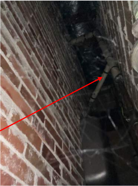
Pipe Insulation in the Pipe Chase between Restrooms
