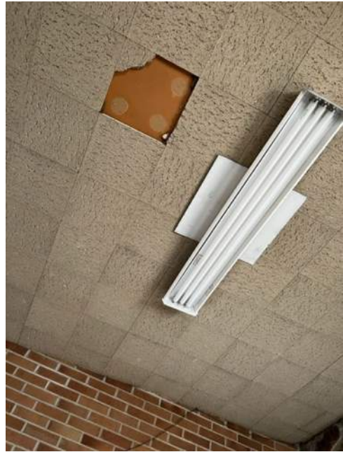
Non-Asbestos Ceiling Tile/Glue Dots with Assumed Pipe Insulation above Plaster Ceiling
