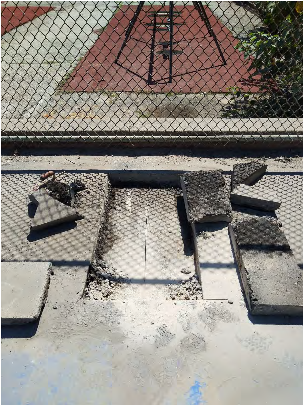
Photo 7: Second test pit on high side of wall: 4 inches of asphalt underlain by a concrete slab. Sawcut concrete slab, thickness unknown (at least 4 inches depth of cut)
