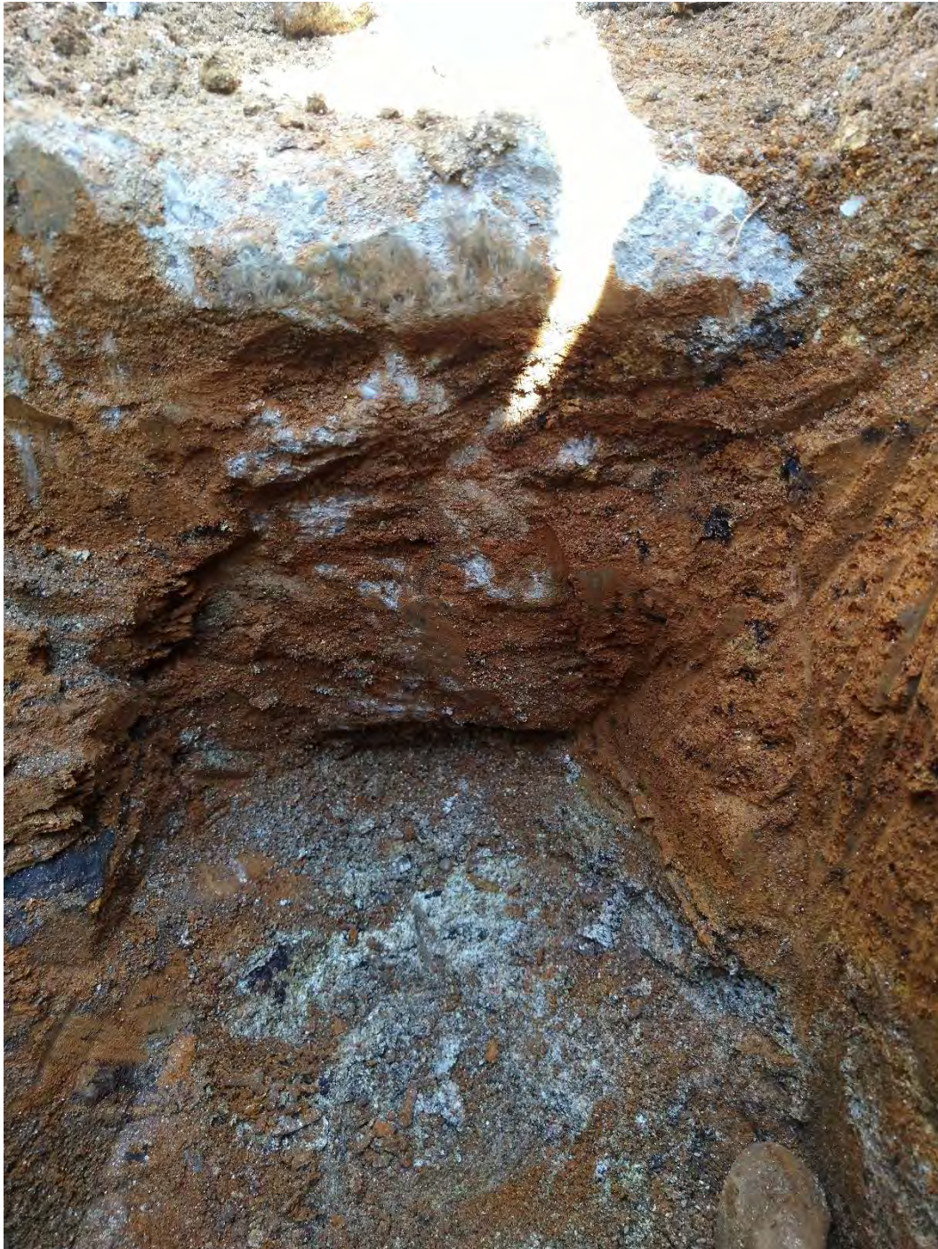
Photo 3: Concrete footing, 12 inches thick and 12 inches protrusion from face of block wall
