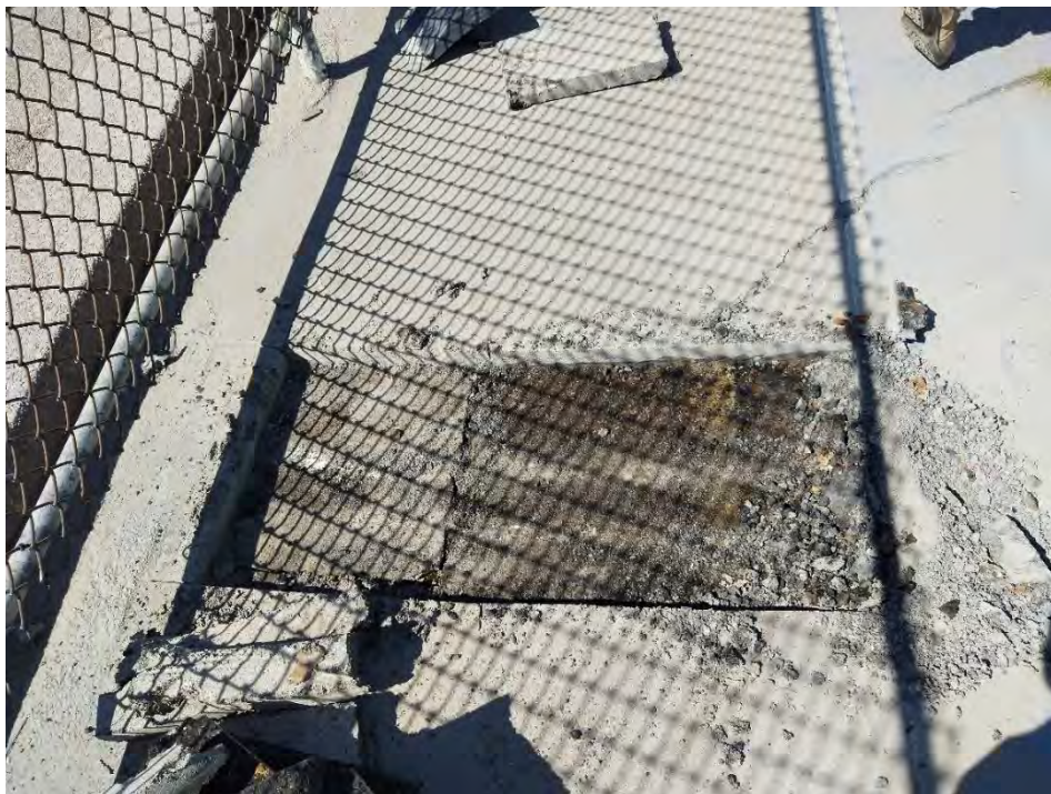
Photo 6: First test pit on high side of wall: 2 inches of asphalt underlain by concrete slab
