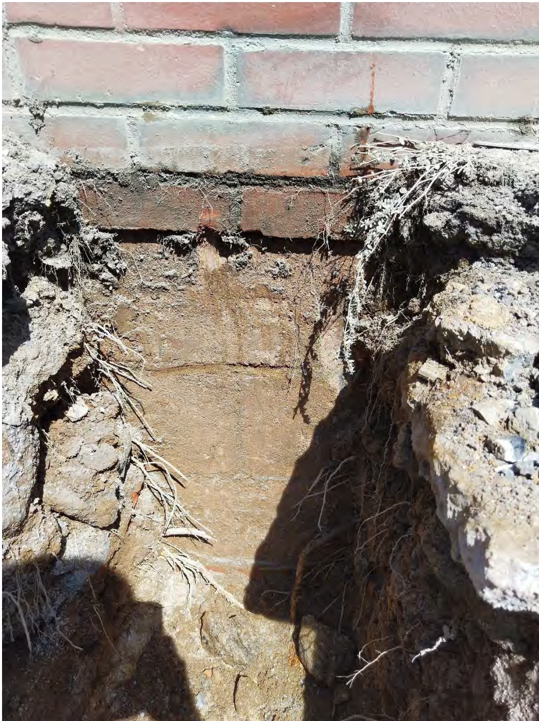
Photo 2: Three courses of CMU block below above-ground brick wall, on top of one course of brick, on top of concrete footing
