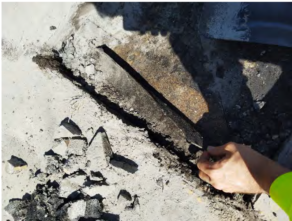
Photo 9: Rubber membrane sandwiched between asphalt (3 inches) and concrete, possible patch over preexisting crack in concrete (suspected location below crack shown in asphalt in previous photo)
