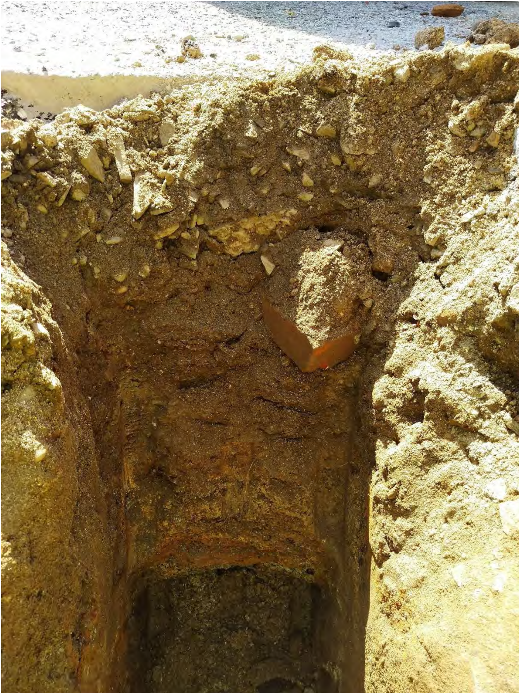
Photo 1: Side of excavation on low side of wall. Brick and fill visible in upper 21 inches.
