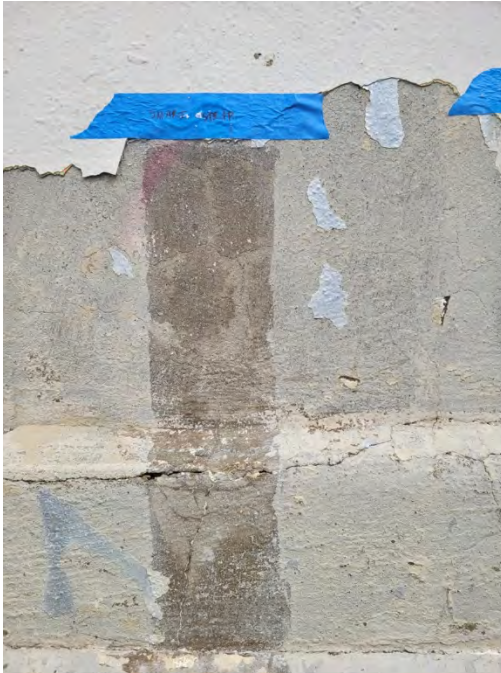
Figure 12. A close-up of the top half of the Smart Strip Pro test location, after testing.
