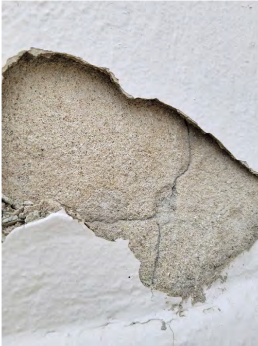
Figure 27. An existing area of deterioration where the portland cement skim coat has detached, exposing the original pale yellow finish coat.
