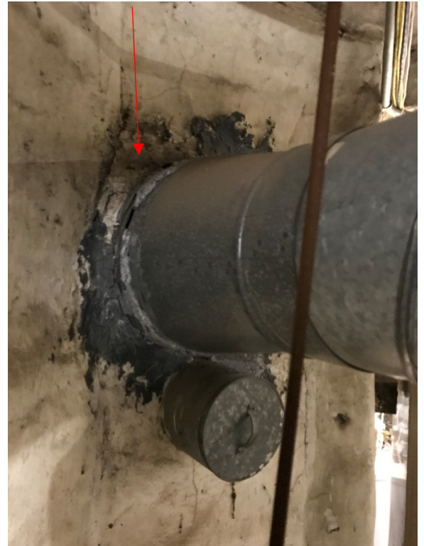
Confirmed asbestos containing White Packing surrounding the Boiler Breeching/Chimney connection point in the Basement Mechanical Room
