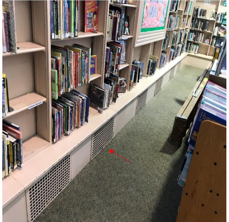
Radiator diffusers incorporated into the First Floor Library Bookshelves – Piping feeding the radiators assumed to be asbestos-insulated
