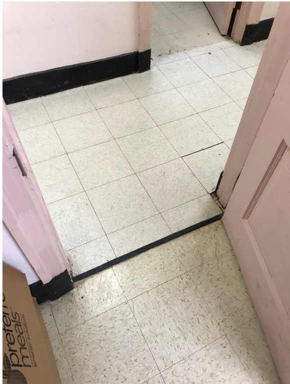
Confirmed asbestos containing 12" x 12" White Floor Tile and associated Mastic throughout the Basement (below non-asbestos VCT in certain locations)
