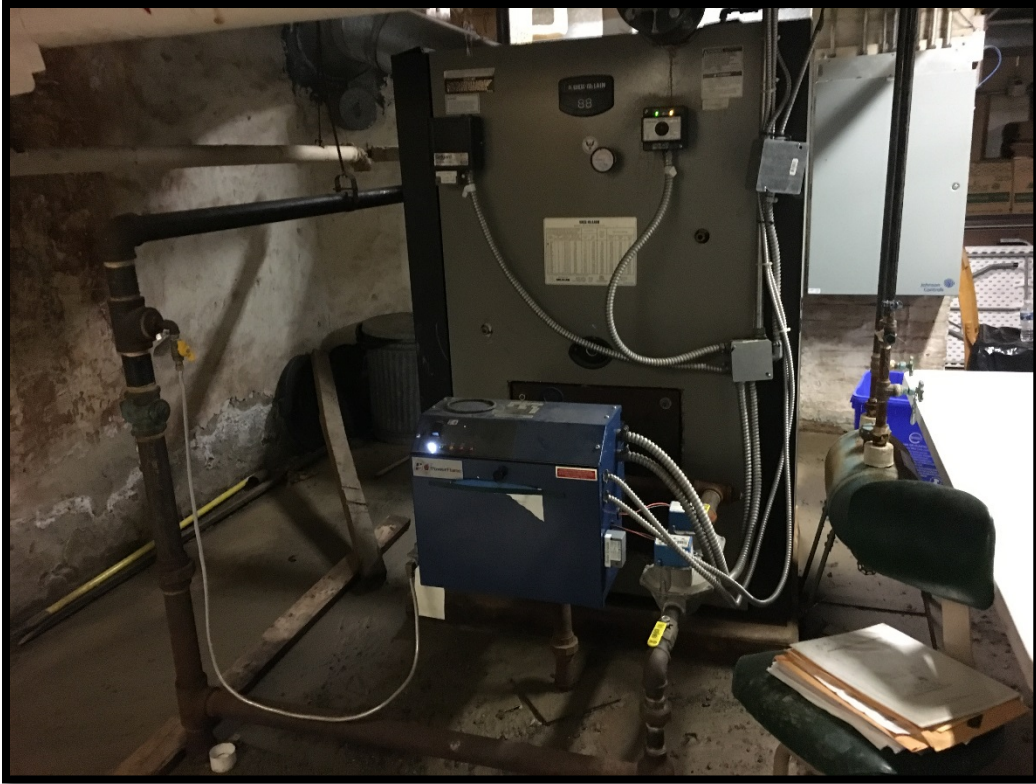
Photograph 9: Boiler room in the basement of McPherson library.
