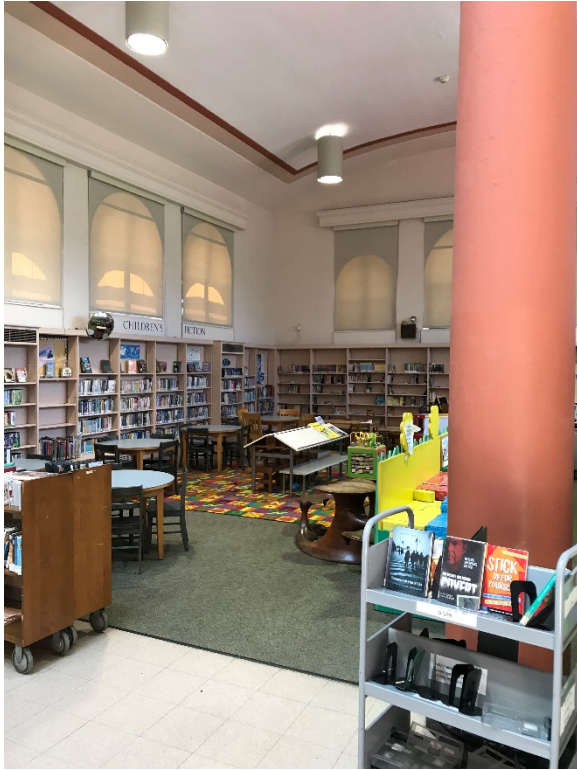
Confirmed asbestos containing 12" x 12" White Floor Tile and associated Mastic throughout the First Floor (below carpeting in certain locations)
