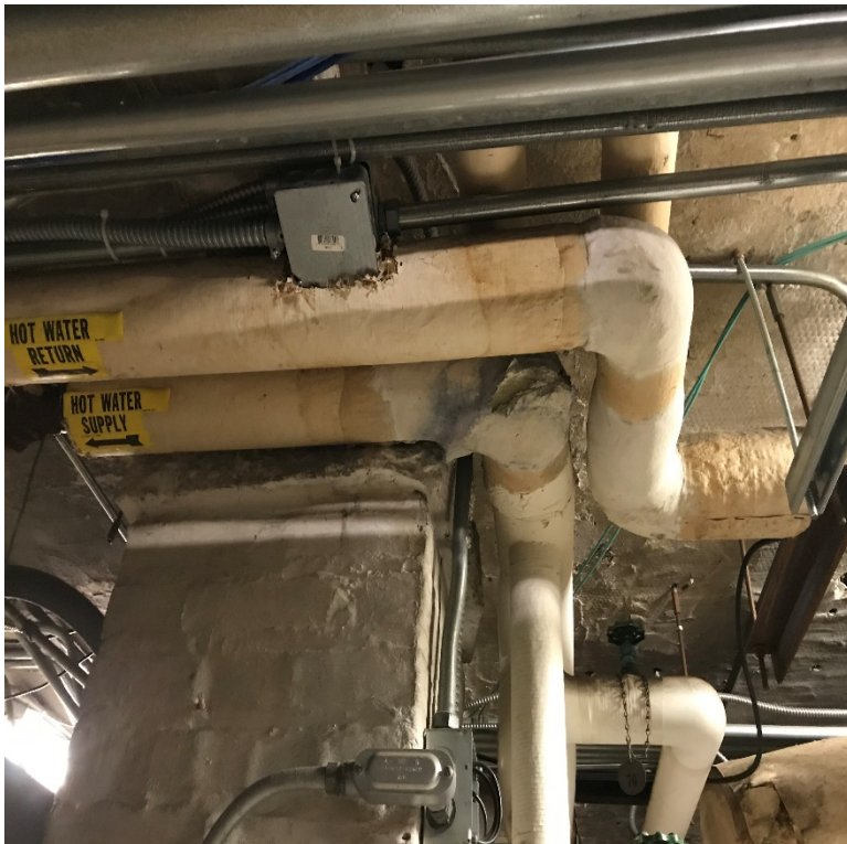
Hard Packed Pipe Fitting Insulation associated with hot water supply and hot water return piping throughout the Basement Mechanical Room verified non-asbestos
