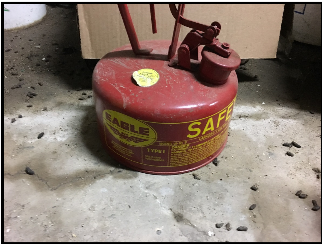
Photograph 12: Gasoline can in the Boiler Room.
