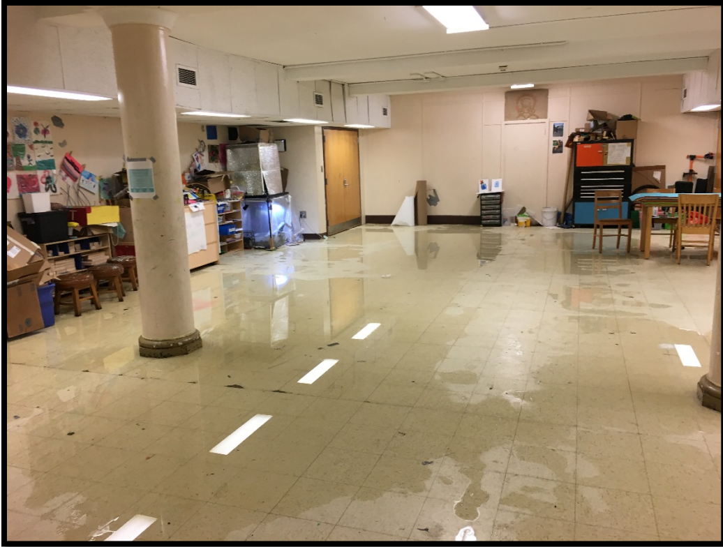
Photograph 13: Flooding in Main Classroom of the Basement.
