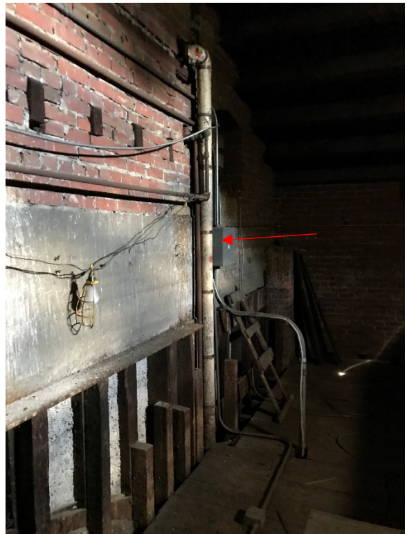
Friable Asbestos Containing Magnesia (MAG) Pipe/Pipe Fitting Insulation identified throughout the Attic
