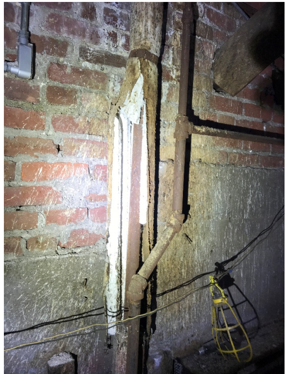
Damaged MAG Pipe Insulation identified in the front portion of the Attic
