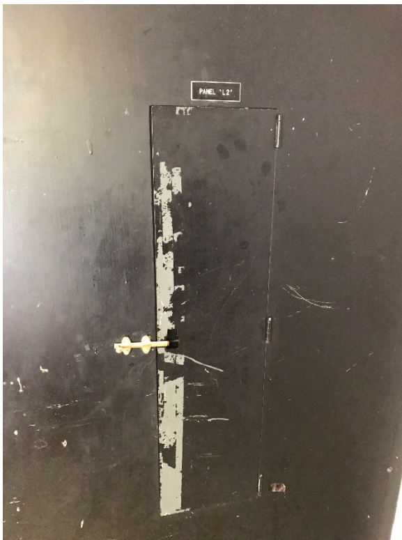
Wire Insulation inside Electric Panels throughout the Building (assumed present; assumed asbestos-containing)
