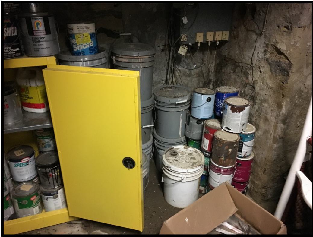
Photograph 11: Miscellaneous cleaning supplies and paint cans in the Boiler Room.
