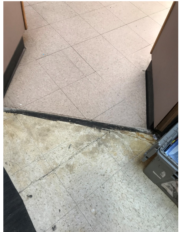
Confirmed asbestos containing 12" x 12" White Floor Tile and associated Mastic throughout the First Floor (below non-asbestos VCT in certain locations)
