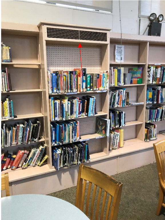
Forced air diffusers incorporated into the First Floor Library Bookshelves
