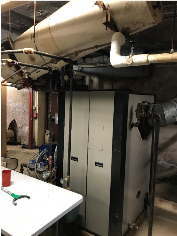
Fiberglass Insulation applied to small Tank above the newer Weil-McLain gas-fired furnace
