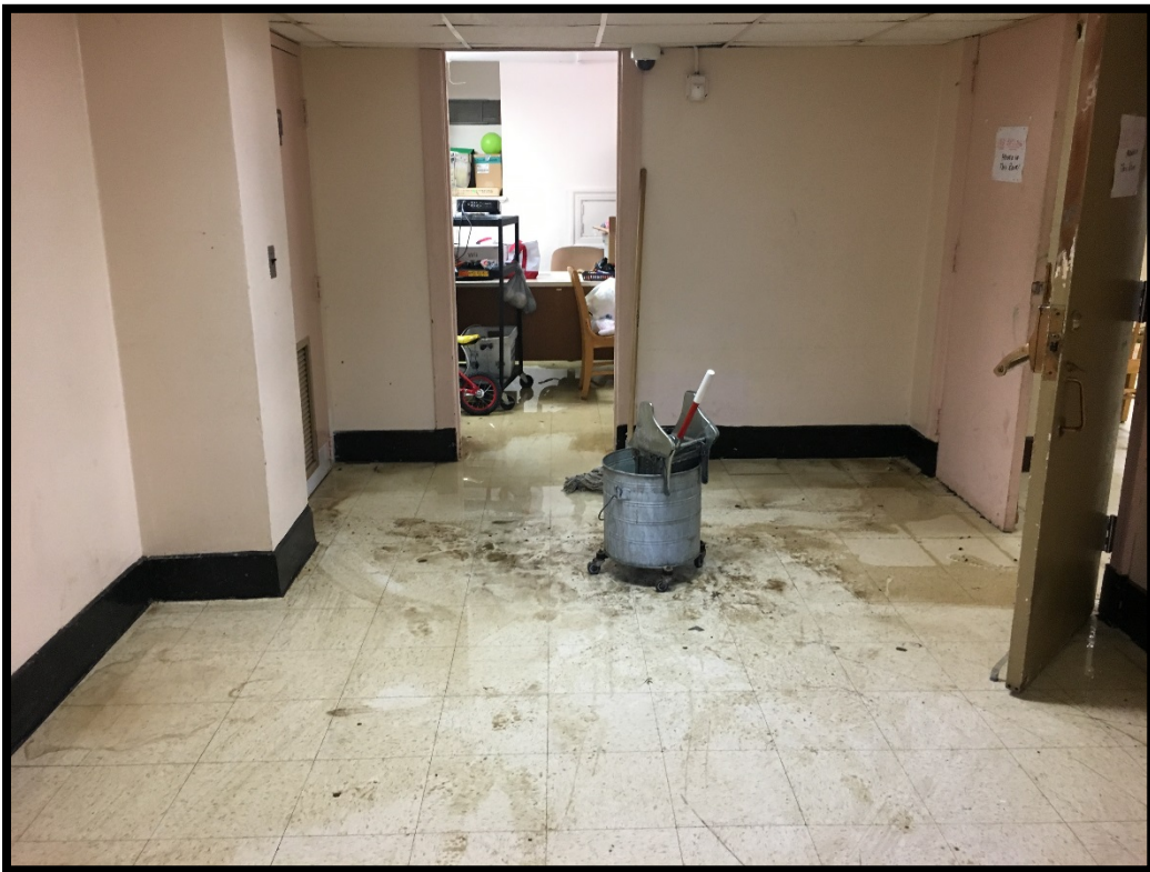
Photograph 14: Flooding in Main Hallway of the Basement.
