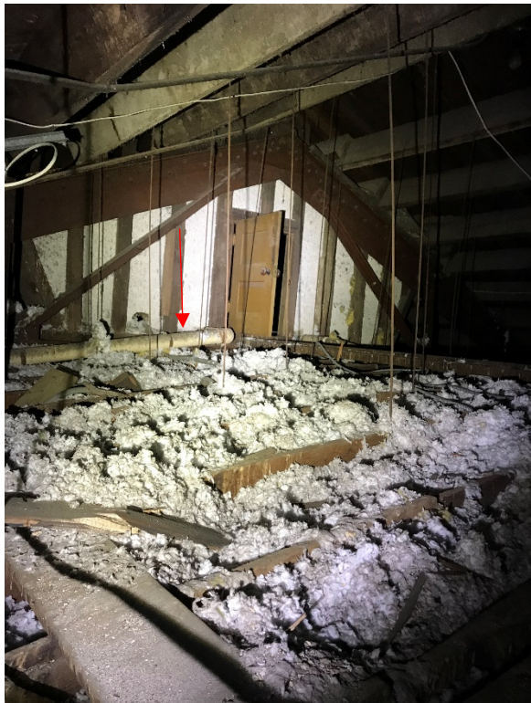
Blown-in Insulation throughout the Attic verified non-asbestos. Friable Asbestos Containing MAG Pipe/Pipe Fitting Insulation identified throughout the Attic
