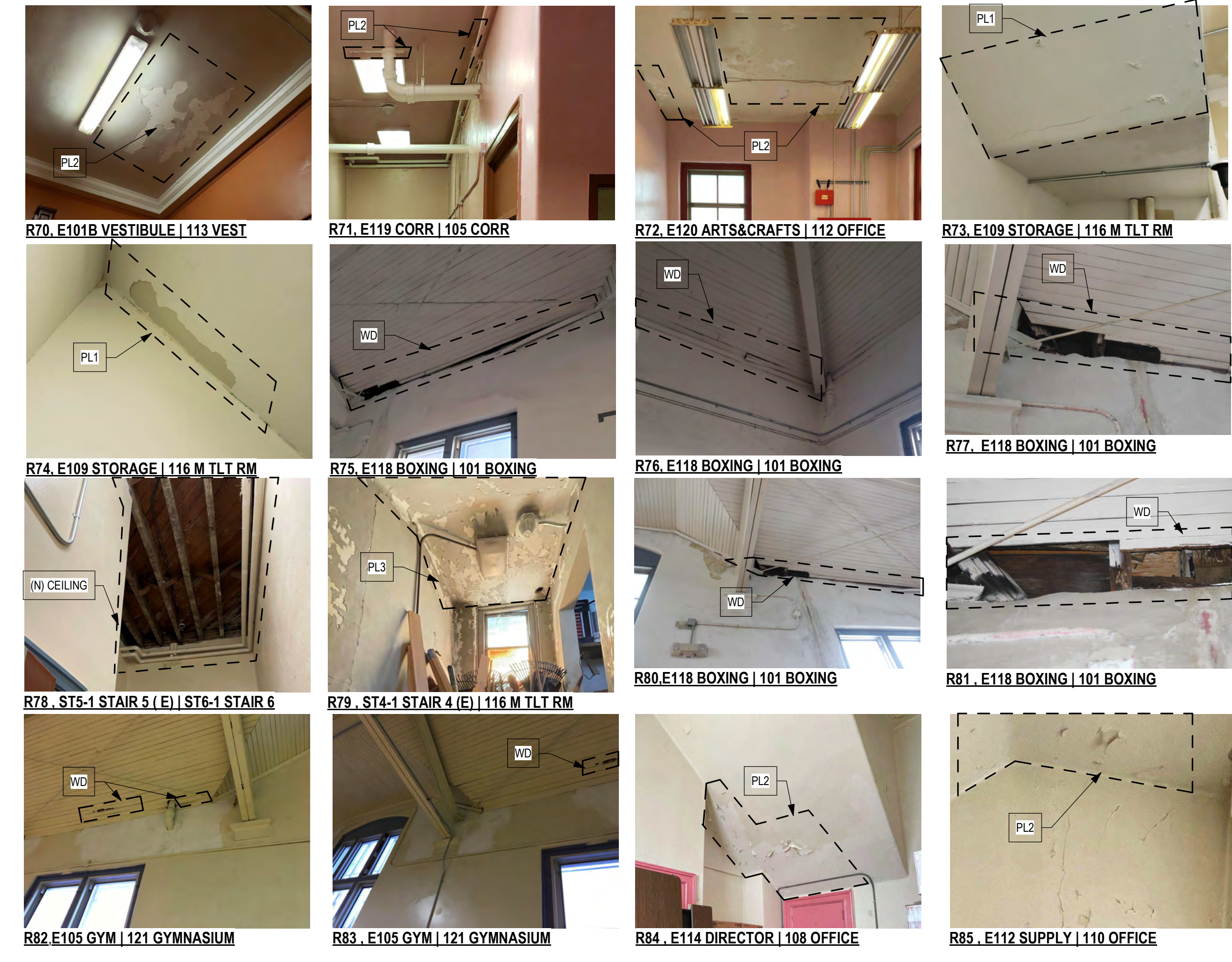
R70. E101B VESTIBULE | 113 VEST R71. E119 CORR | 105 CORR R72. E120 ARTS&CRAFTS | 112 OFFICE R73. E109 STORAGE | 116 M TLT RM R74. E109 STORAGE | 116 M TLT RM R75. E118 BOXING | 101 BOXING R76. E118 BOXING | 101 BOXING R77. E118 BOXING | 101 BOXING R78. ST5-1 STAIR 5 (E) | ST6-1 STAIR 6 R79. ST4-1 STAIR 4 (E) | 116 M TLT RM R80. E118 BOXING | 101 BOXING R81. E118 BOXING | 101 BOXING R82. E105 GYM | 121 GYMNASIUM R83. E105 GYM | 121 GYMNASIUM R84. E114 DIRECTOR | 108 OFFICE R85. E112 SUPPLY | 110 OFFICE
