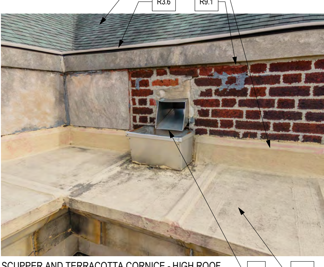
SCUPPER AND TERRACOTA CORNICE - HIGH ROOF NOTE: REMOVE ALL UPPER LEVEL TERRACOTA CORNICE PIECES, INCLUDING STEEL SUPPORTS. SEE STRUCTURAL DRAWINGS.
