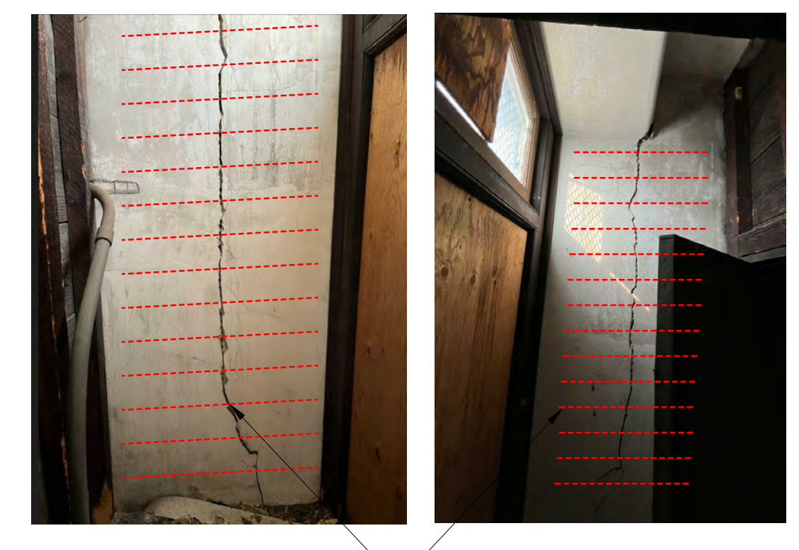
EXPOSE BRICK. PROVIDE 3/8" X 12" BRICK HELICAL TIES THROUGH MORTAR JOINTS AT 8' O.C., FULL HEIGHT OF WALL CRACKS
