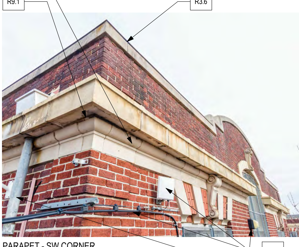
PARAPET - SW CORNER NOTE: REMOVE ALL SECURITY GRATINGS AT ALL WINDOWS. PATCH MASONRY AS REQUIRED PRIOR TO INSTALLATION OF NEW WINDOWS.
