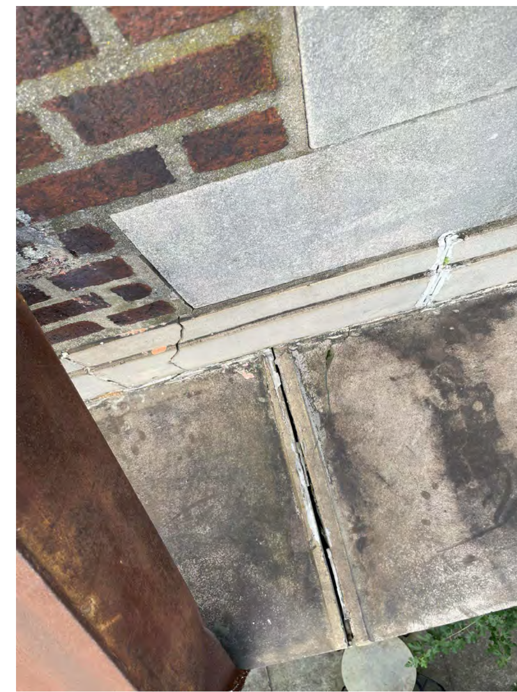
8 ROOF CONDITION - TERRACOTTA CORNICE
