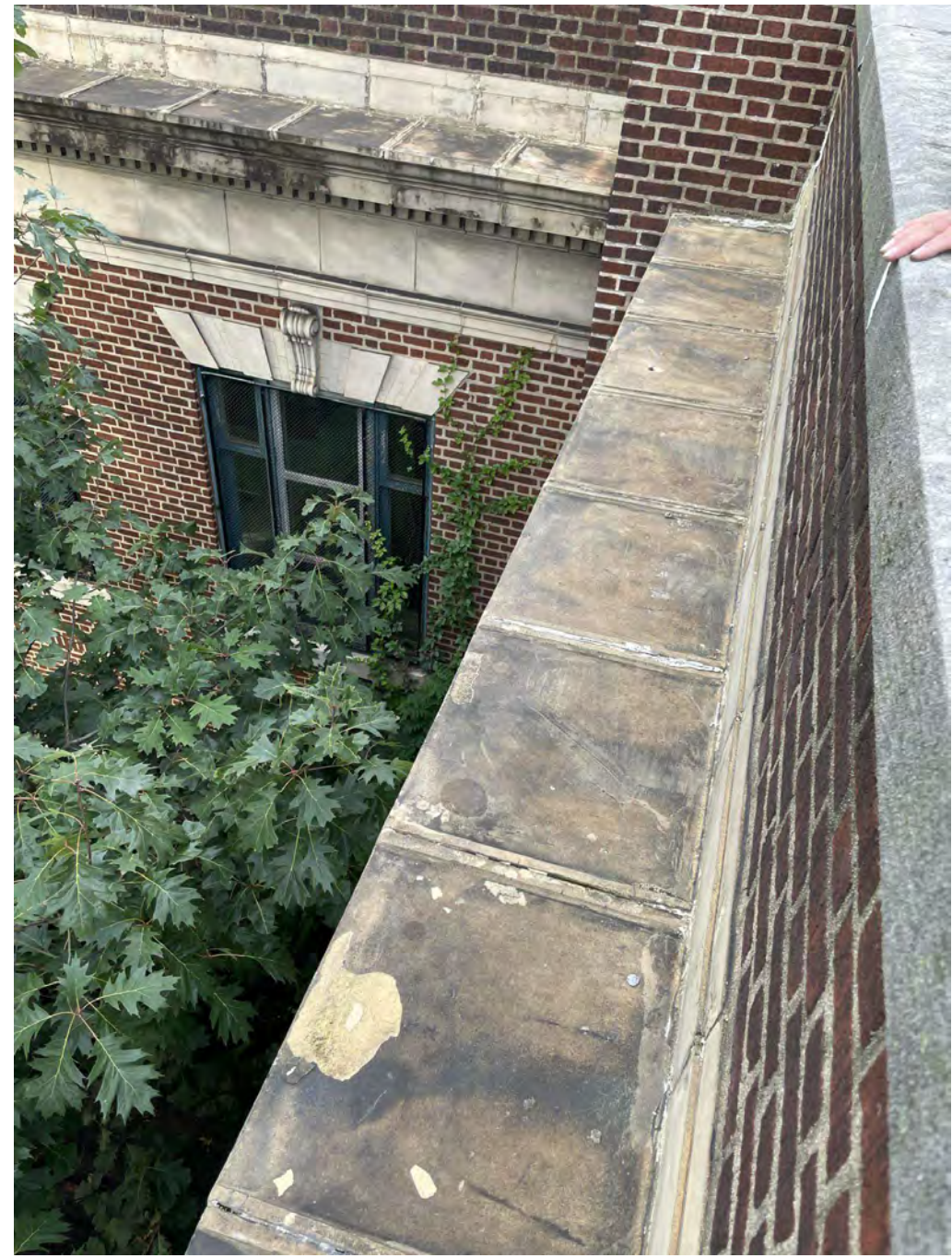
5 ROOF CONDITION - TERRACOTTA CORNICE
