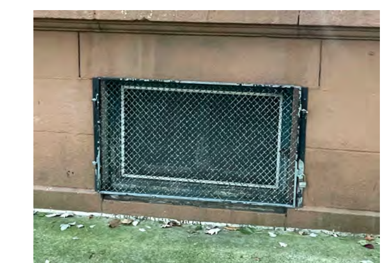
3 NORTH ELEVATION L.L. WINDOW CONDITION TYP 023 SEE SCOPE OF WORK WW AND WS
