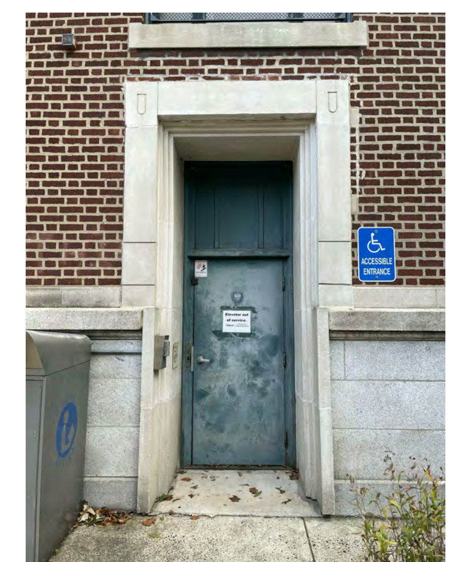
3 ELEVATOR ENTRANCE DOOR
