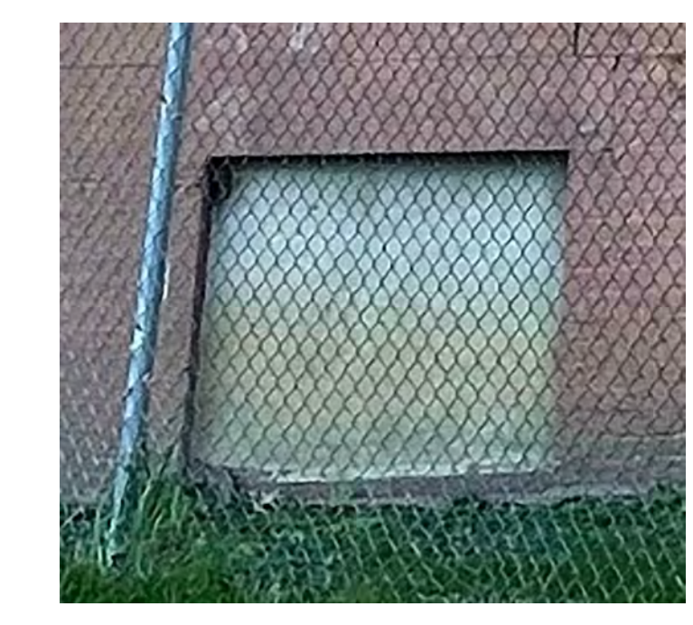
4 EAST L.L. WINDOW CONDITION 2 - MASONRY INFILL TYP 017, 018, 019 SEE SCOPE OF WORK M-1
