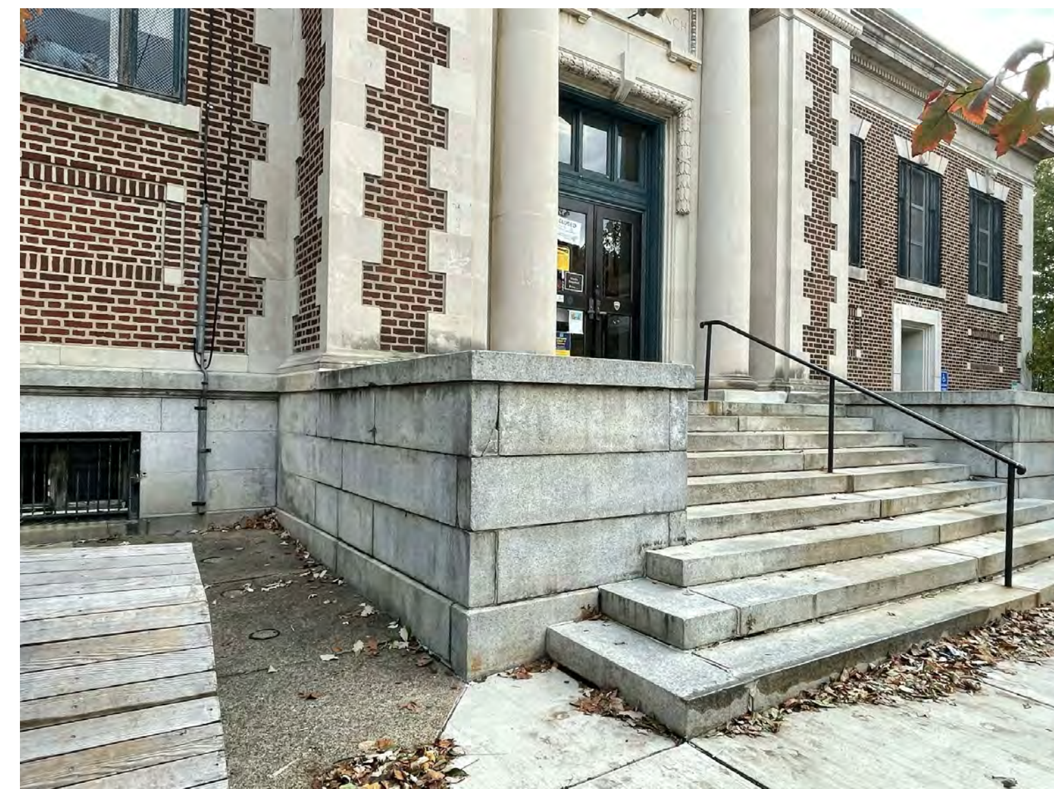
5 MAIN ENTRANCE STAIR CONDITION
