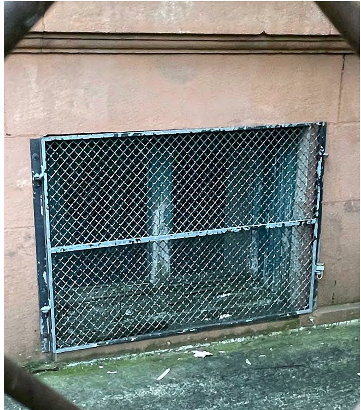
6 LOWER LEVEL WINDOW CONDITION TYP 021,022 SEE SCOPE OF WORK WW AND WS
