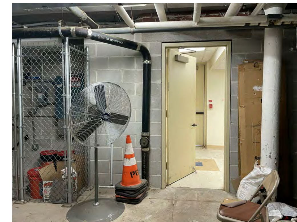
6 BOILER ROOM - LOWER LEVEL
