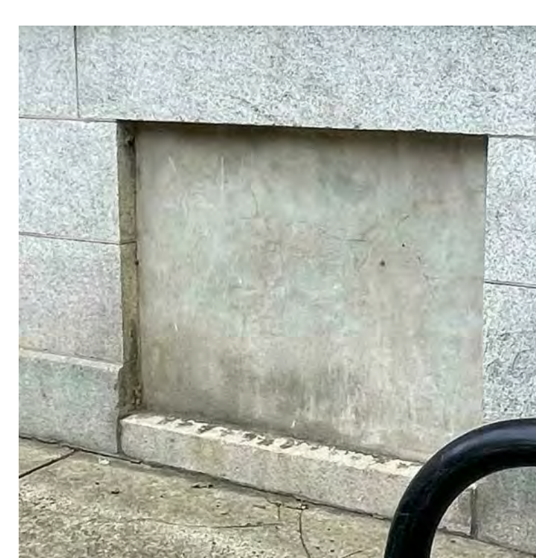
9 L.L WINDOW CONDITION - WDW 004
