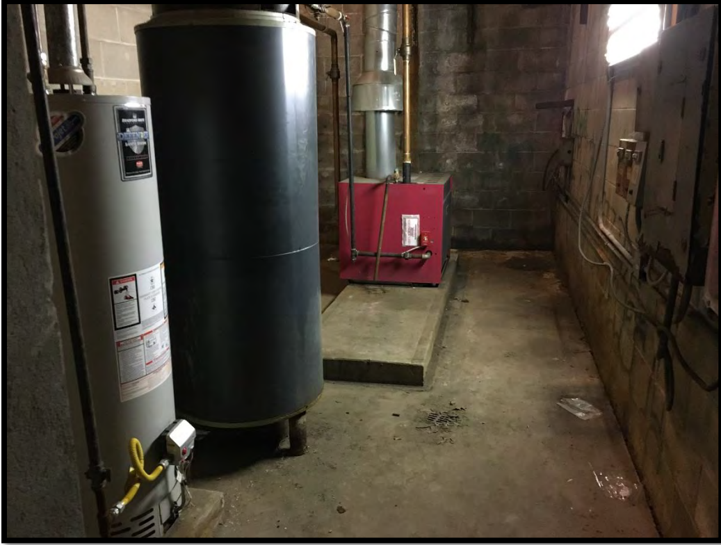
Photograph 21: Boiler room in the basement.
