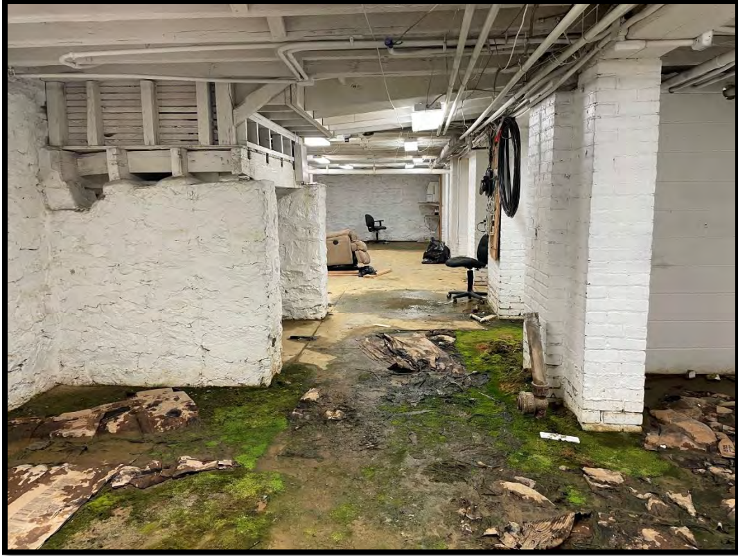
Photograph 27: Basement of Annex with pool of water.
