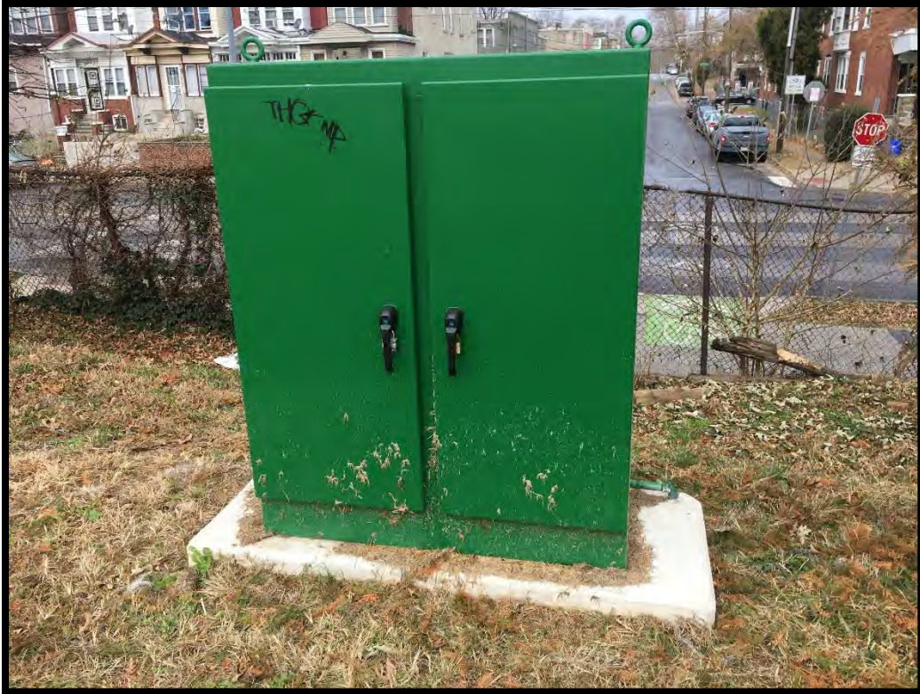
Photograph 15: Meter for field lights observed west of the baseball fields of the Property.
