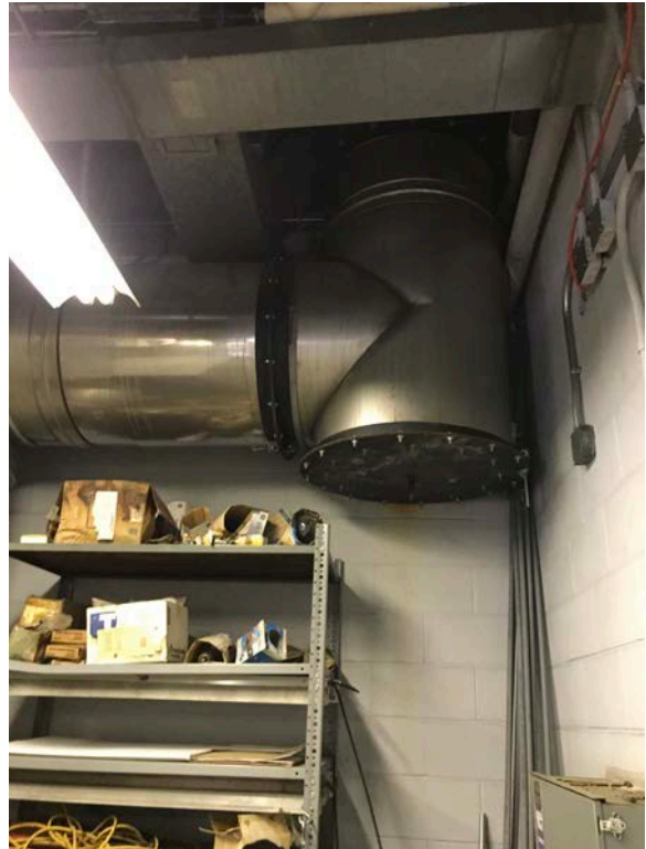
Boiler Breeching Gaskets (assumed present; assumed asbestos-containing)
