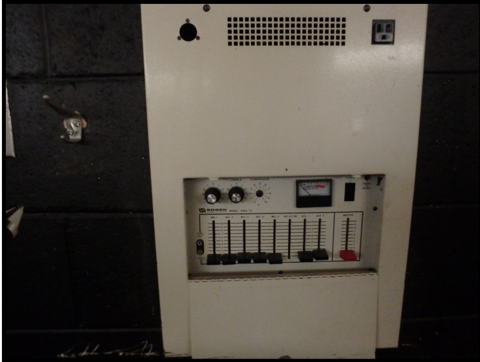
Photograph 17 – Control panel in gymnasium
