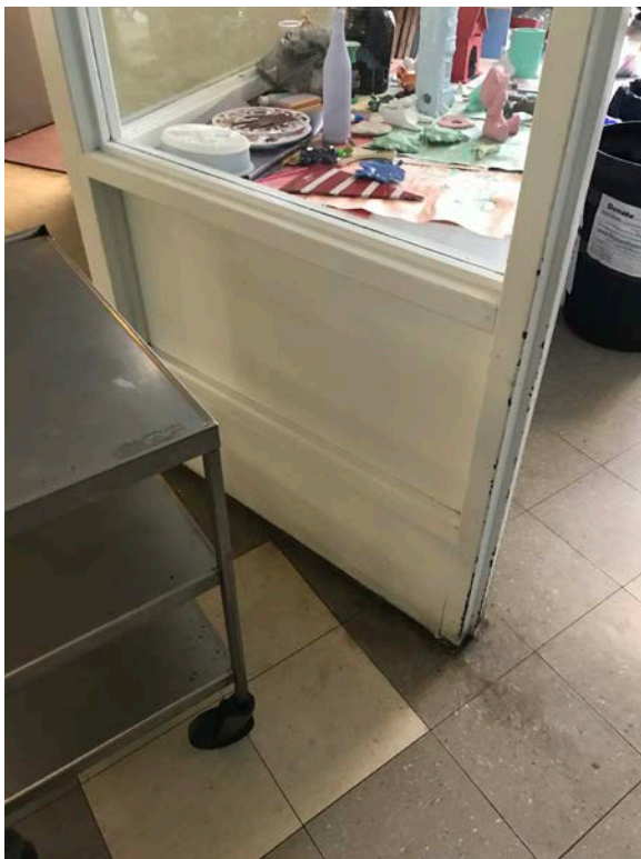
Insulation inside Metal Panel associated with Storefront Window at Entrance to Art Room (assumed present; assumed asbestos-containing)
