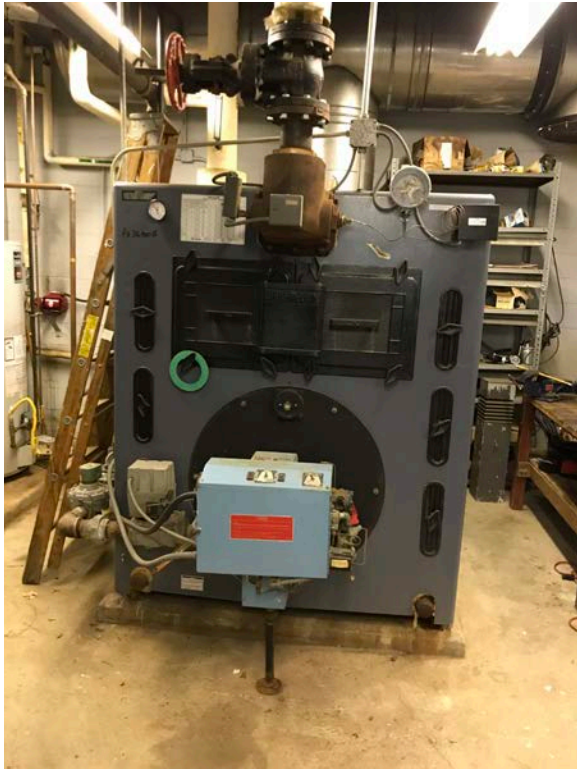
Weil-McLain 94 Series Sectional Boiler (internal materials assumed asbestos-containing)
