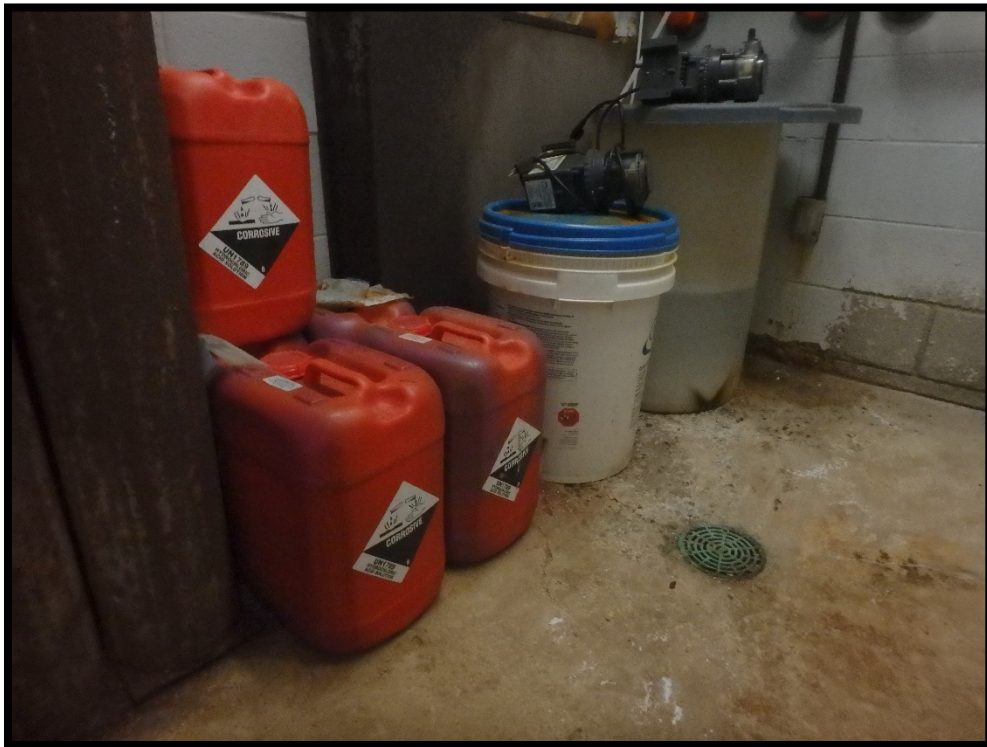
Photograph 12 – Pool chemicals in room adjacent to utility room in pool area.
