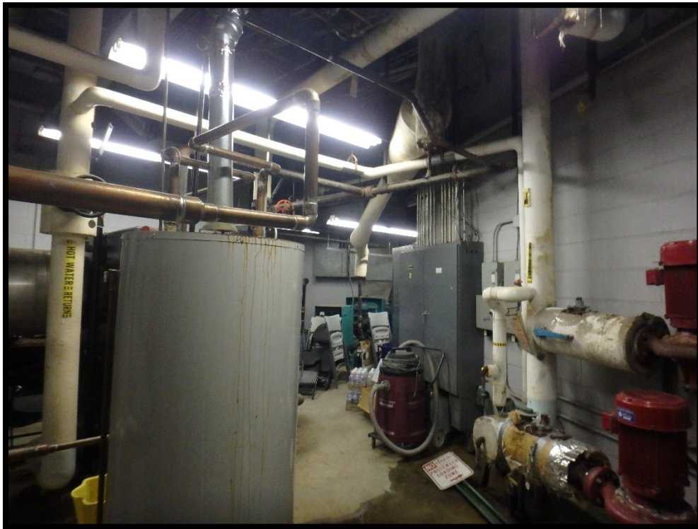
Photograph 14 – Mechanical room with boilers, HVAC, transformers and control panels.
