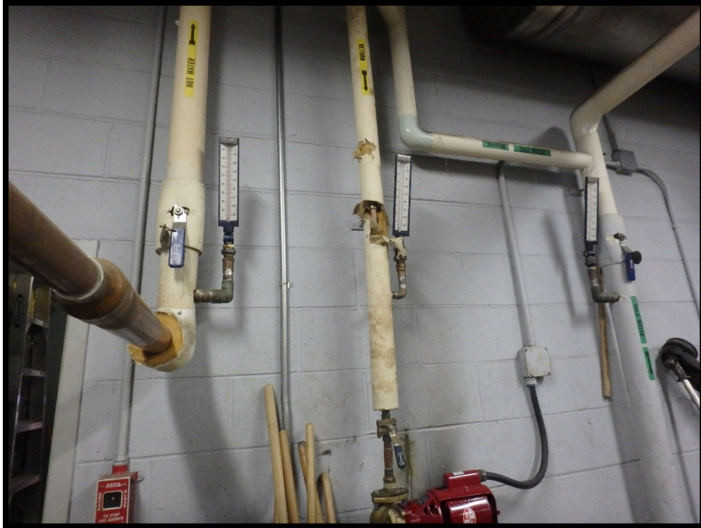
Photograph 15 – Thermometers monitoring pipes in mechanical room.
