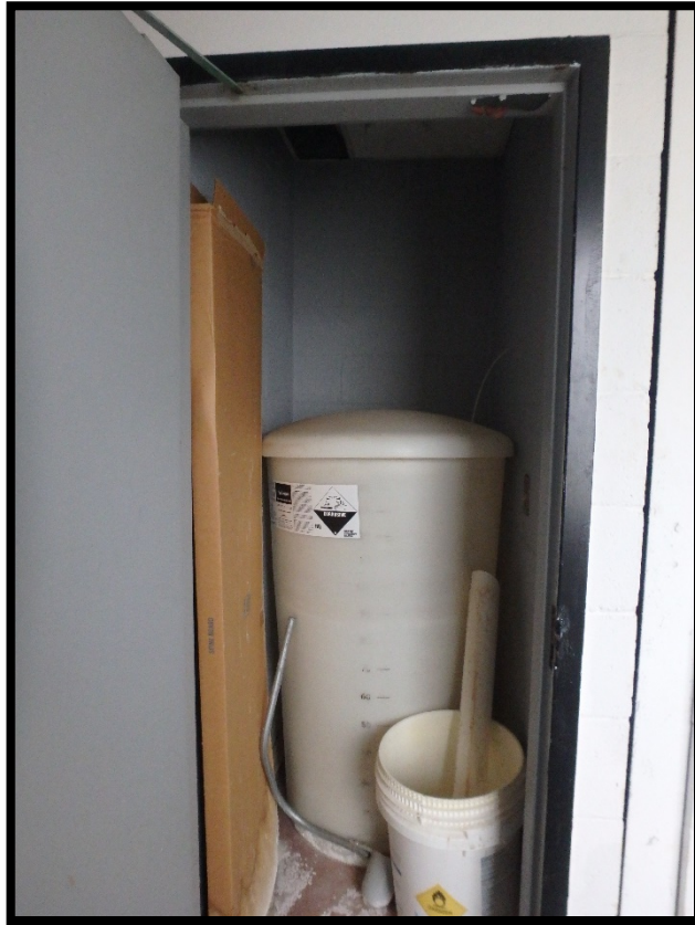
Photograph 13 – Pool chemicals in storage closet in hallway in pool area.
