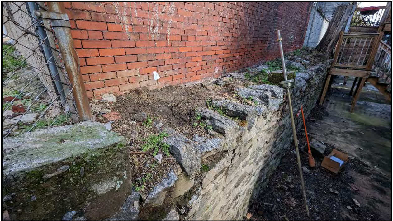
Photo 4: GF-3 looking northeast towards stone masonry wall and garage on adjacent property.
