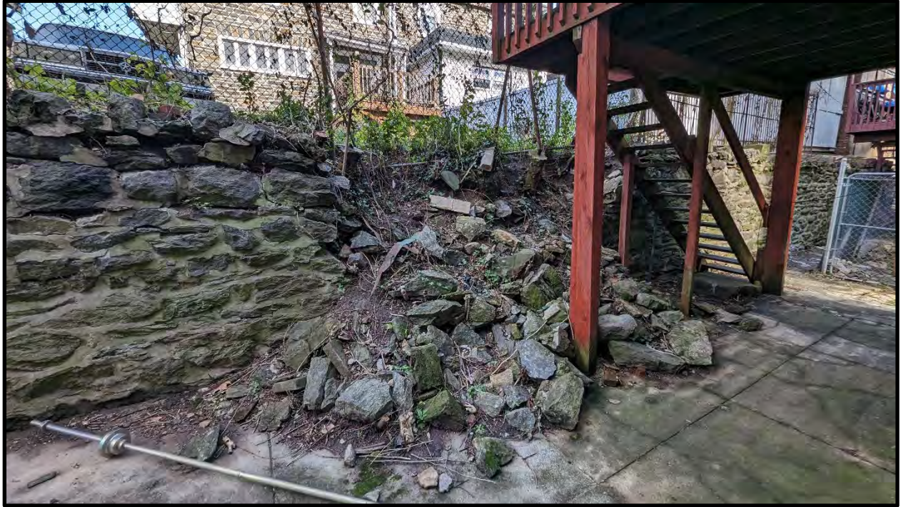
Photo 5: Collapsed stone masonry wall between GF-3 and GF-5 looking northeast
