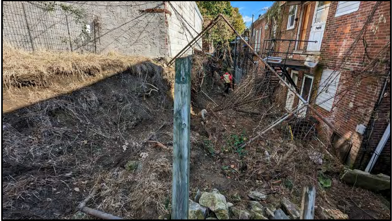
Photo 9: GF-5 looking east down alley showing soil failure and collapsed stone masonry wall
