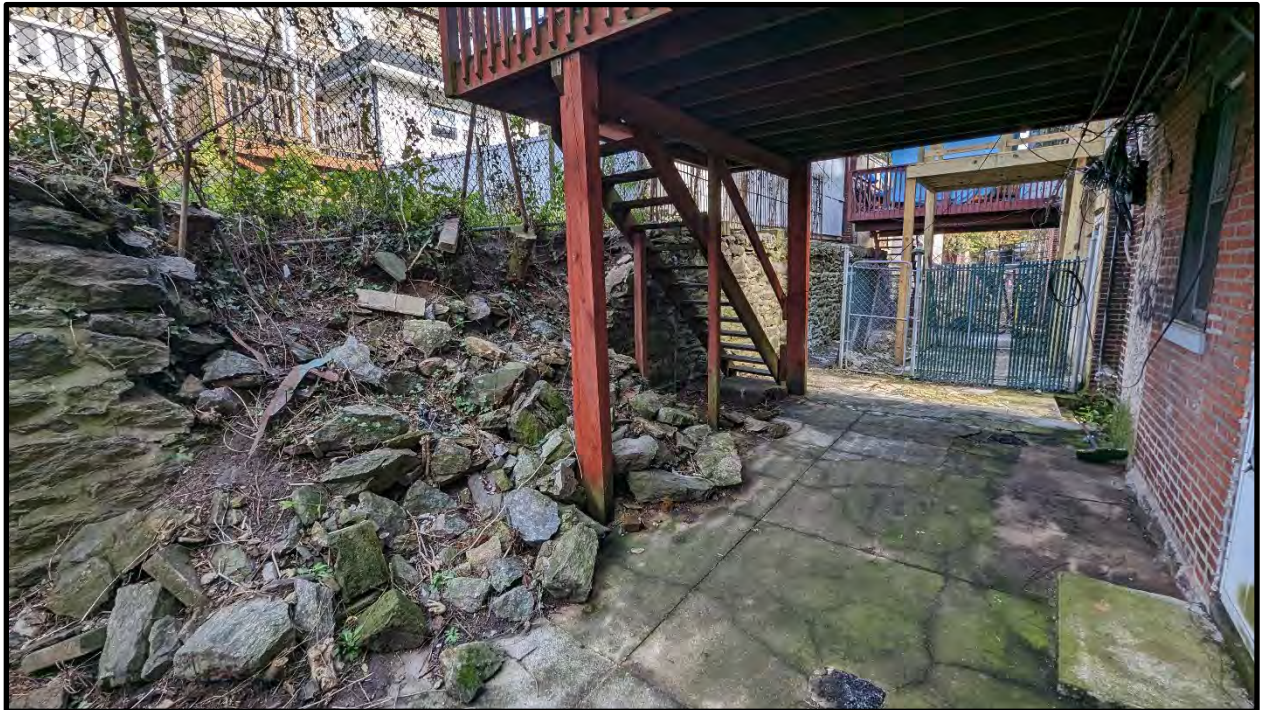
Photo 6: Collapsed stone masonry wall between GF-3 and GF-5 looking east
