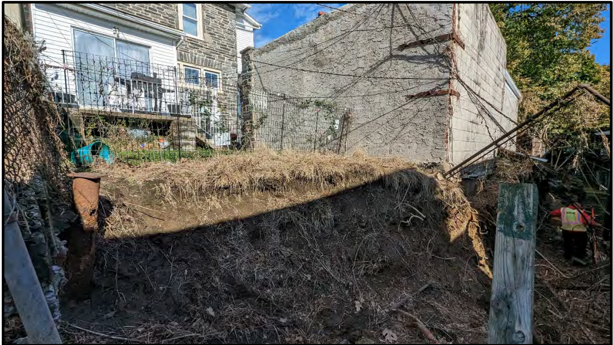
Photo 8: GF-5 looking north towards collapsed stone masonry wall, soil failure, and garage on adjacent property
