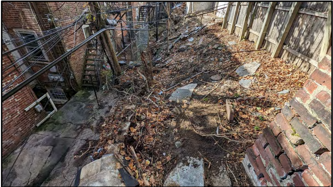
Photo 10: GF-6 looking west showing failing stone masonry retaining wall and damaged utilities
