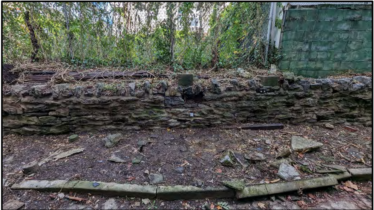
Photo 2: GF-2 looking north towards deteriorating stone masonry wall
