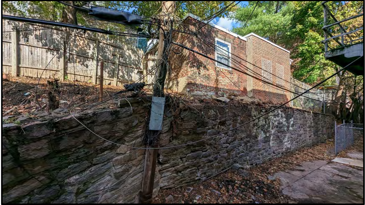
Photo 11: GF-6 looking northeast showing failing retaining wall leaning against utility pole
