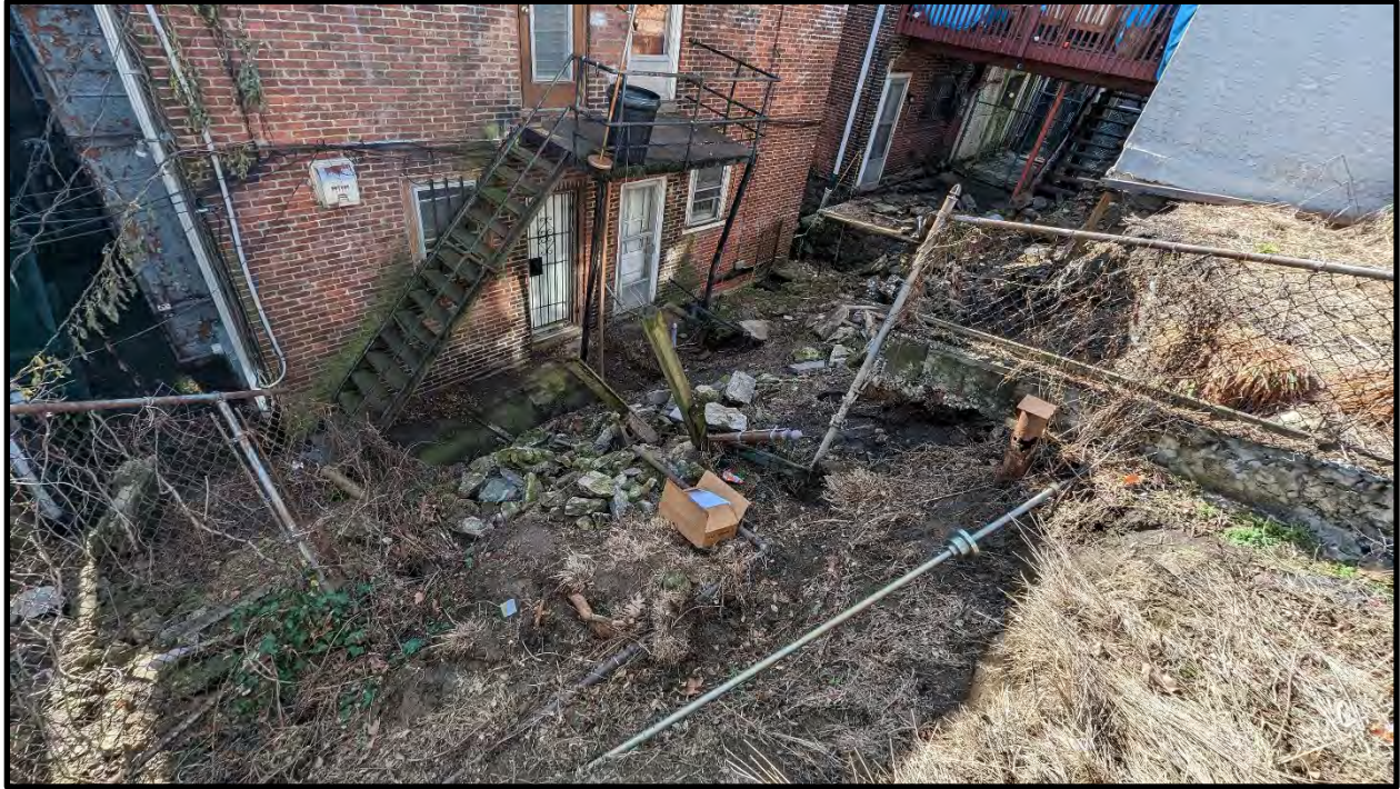
Photo 7: GF-5 looking south towards collapsed stone masonry wall, damaged utilities and stairs
