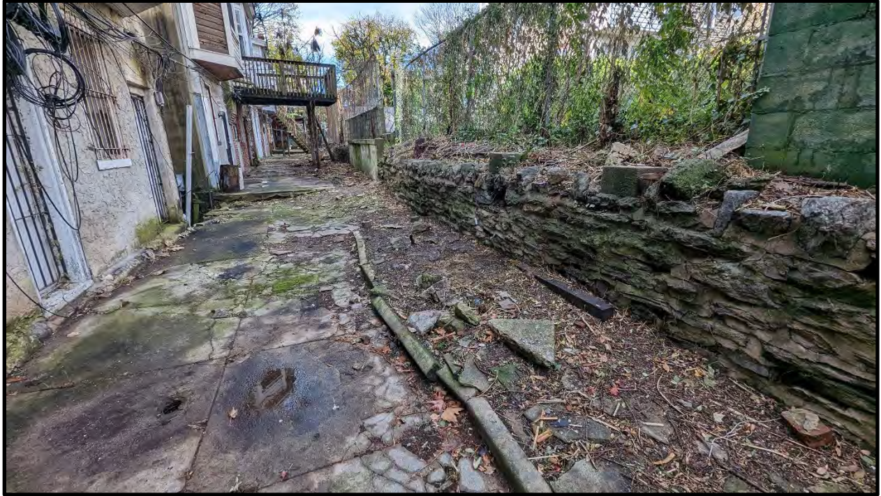
Photo 3: GF-2 looking east towards deteriorating stone masonry wall
