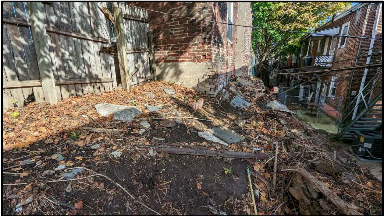
Photo 12: GF-6 looking east showing conditions above wall, repairs made to adjacent structure
