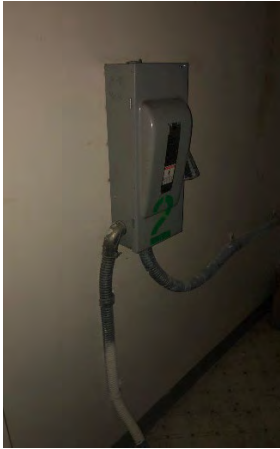
First floor elevator room panel.
