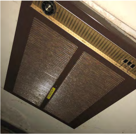
First floor corridor heater at main entrance.
