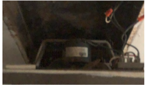
First floor corridor heater at main entrance.
