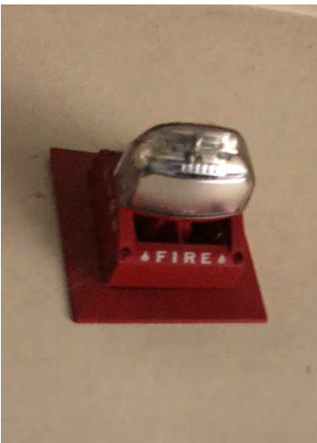
First floor fire alarm strobe.
