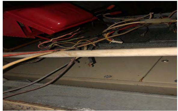
Unit 1a electric wiring next to indoor unit.
