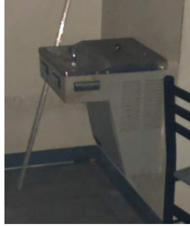
First floor water fountain in management office.
