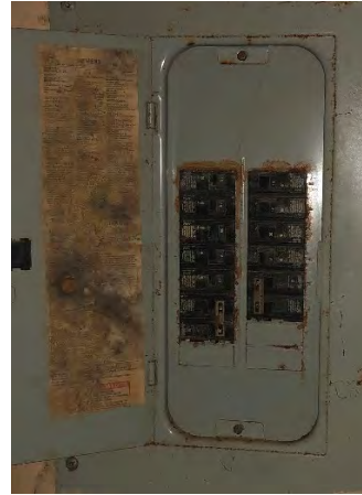
Unit 1a electric panel.
