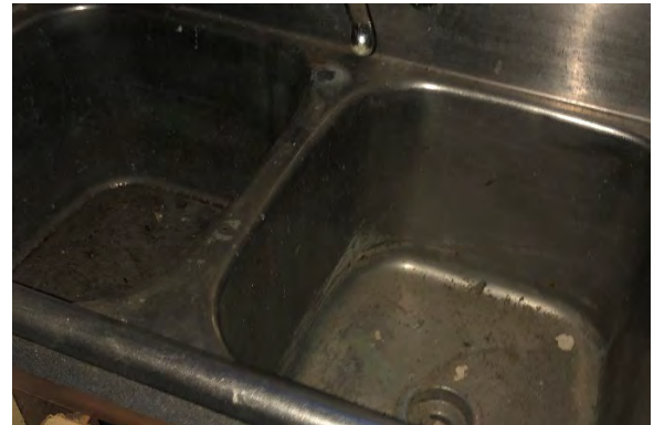
First floor management room sink/faucet.
