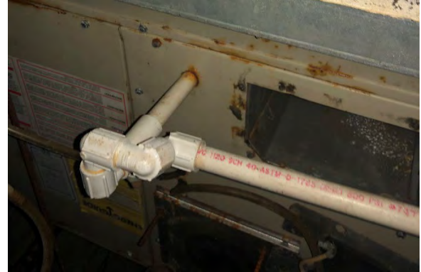
Unit 1a indoor gas unit.
