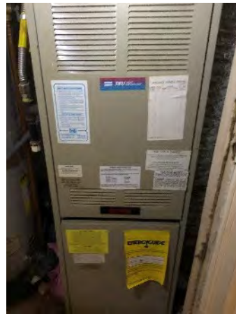
Gas fired furnace in good condition.
