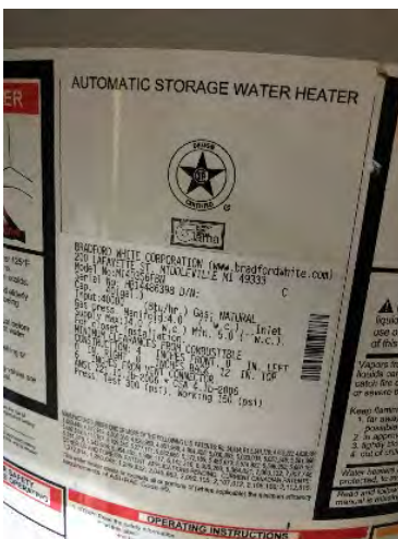
Hot water heater label.
