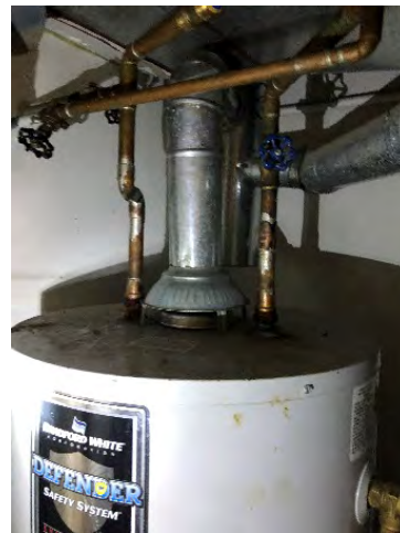
Top of hot water heater in good condition.
