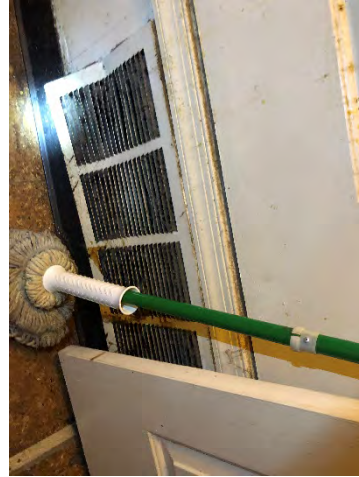
Return vent that needs to be replaced.
