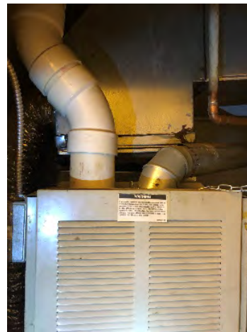
Gas fired furnace in good condition.
