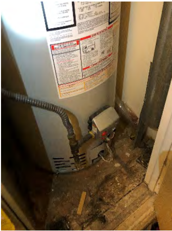
Gas hot water heater.
