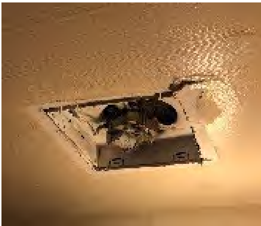
Bathroom exhaust fan (not working).
