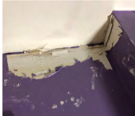
Master bedroom leak damage.
