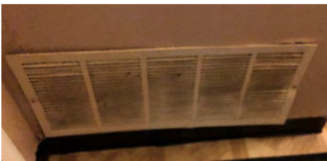
Return grill; only one that might need replacing.
