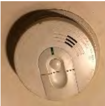
Hard wired fire alarm.
