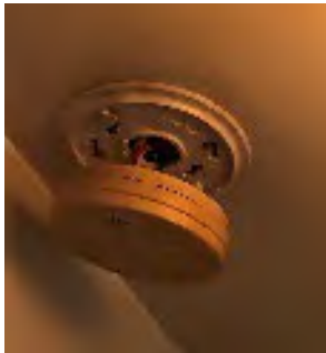
Hard wired fire alarm.
