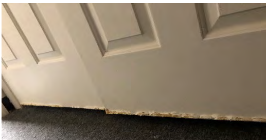
Water damage from laundry room.
