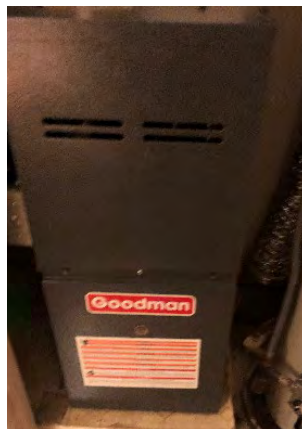
Gas fired furnace and hot water heater.
