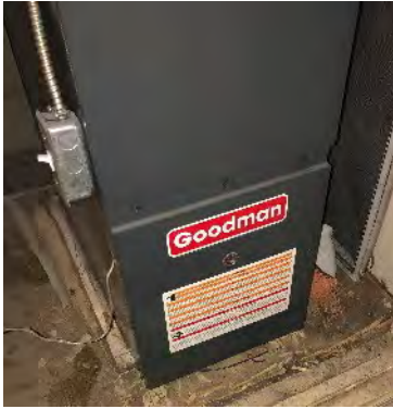
Brand new gas fired furnace.
