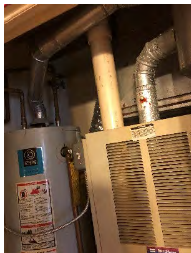
Gas hot water heater and furnace
