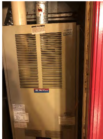
Gas fired furnace working well
