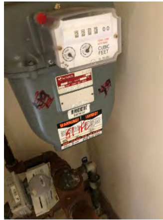
Gas and water meter
