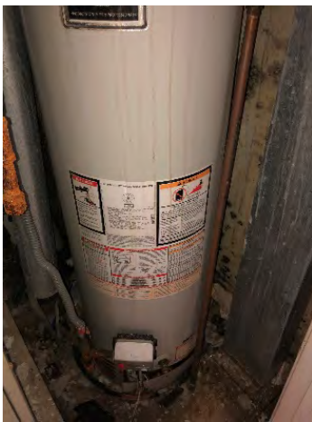
Gas hot water heater
