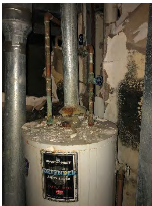
Top of hot water heater
