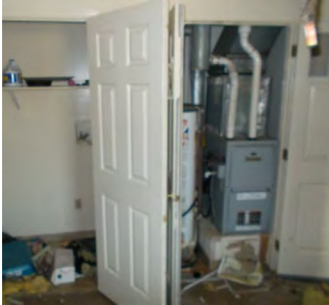
Depicts view of installed hot air furnace and water heater as well as washer/dryer closet facing the kitchen area.
