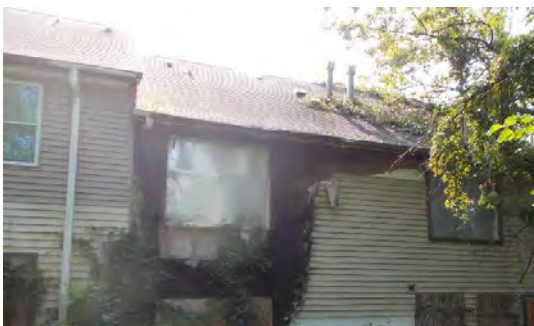
View of fire damage at the rear and damaged roof of units 45 and 47.
