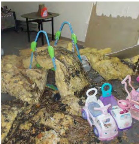
View of gypsum wallboard and insulation that has fallen from the roof trusses above.
