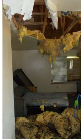
View looking into bedroom. View of collapsed ceiling, wallboard and insulation.
