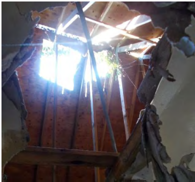
View of damaged ceiling and roof open to elements.
