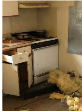
Kitchen gas stove
