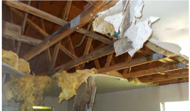
Depicts view of ceiling at living area. View is looking towards front of dwelling.
