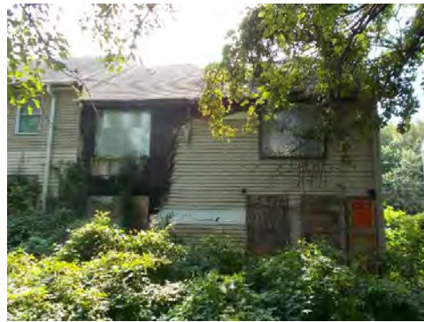
Overall view at the rear of units 45 and 47. Note visible fire damage at rear of unit 45.
