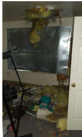
View looking into master bedroom from hallway. Evidence of additional ceiling collapse visible.
