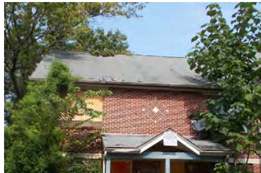
View of fire damage on the roof at the front of units 45 and 47.
