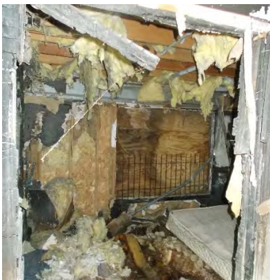
View inside bedroom. Note substantial damage from fire. However, wood framing appears to be in tact.
