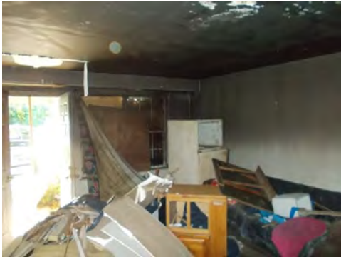
View looking at living room. Unit had evidence of previous fire damage.
