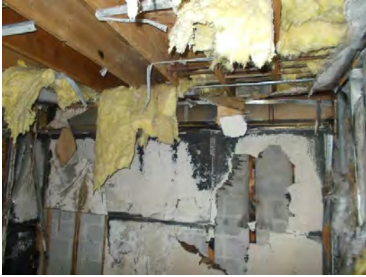
View of damaged area along party wall. Note no damage to the masonry party wall was evident.
