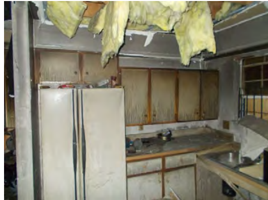
Additional view of kitchen. Depicts damaged ceiling.
