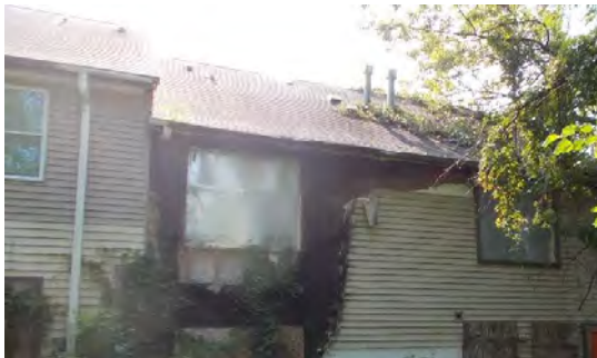
View of fire damage at the rear and damaged roof of units 45 and 47.
