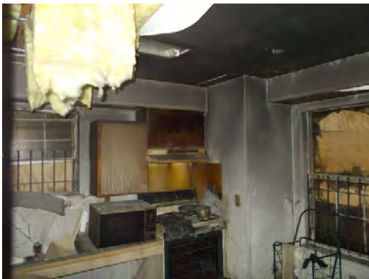
View looking at kitchen. Note window to the right of photo is looking towards rear yard.
