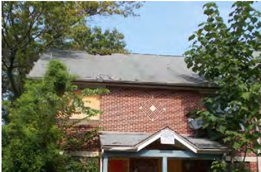
View of fire damage on the roof at the front of units 45 and 47.
