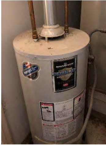
Hot water heater fairley.
