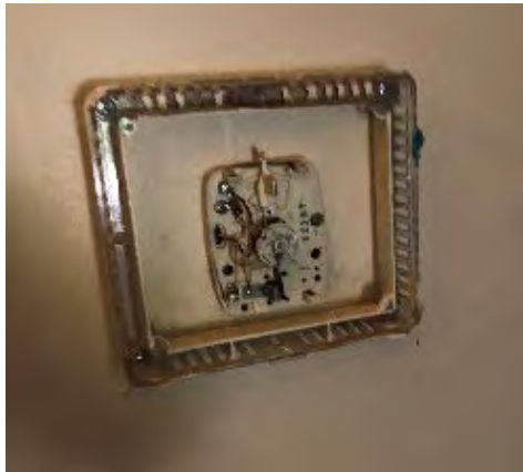
Thermostat with exposed wire.
