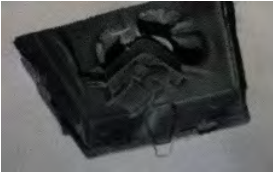
Exhaust fan not working
