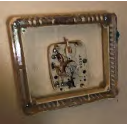
Thermostat with exposed wire
