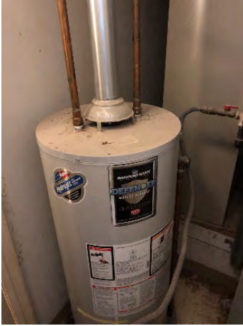
Hot water heater fairley
