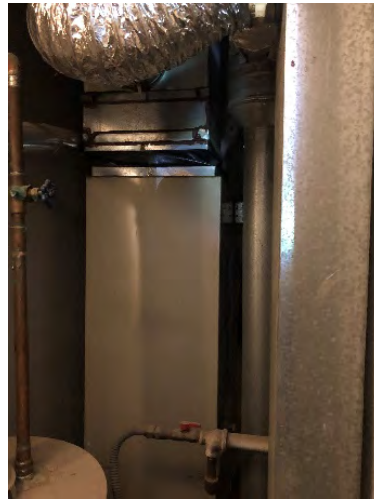
Side of furnace
