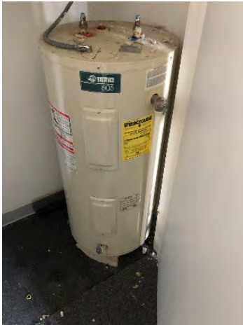
Main hot water heater in master bedroom.
