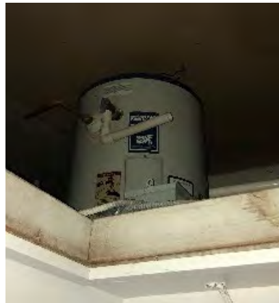
Small hot water heater in master closet ceiling.
