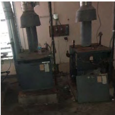
Boiler room furnaces (old).
